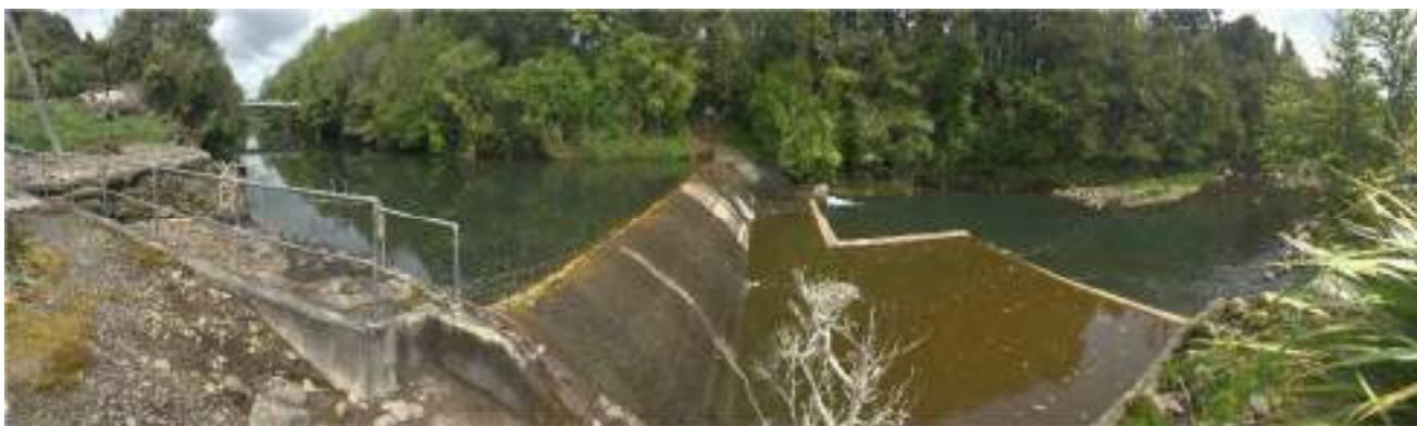
Figure 3.2 The Manganui Weir, wide angle view from right bank. Tariki Road bridge visible on the left of the photo (photo credit: Trustpower)
