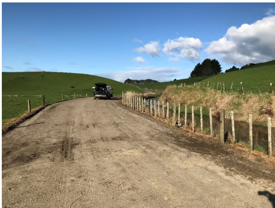
Photo 4: View downstream from CH 1830m (June 2020). The freeboard at the time of the inspection was estimated to be 400mm on the true left bank. The paddock to the left of the farm track is lower than the track. The low point in the track is evident in the lower to centre part of the photo. The vehicles are parked at the high point on the track.
