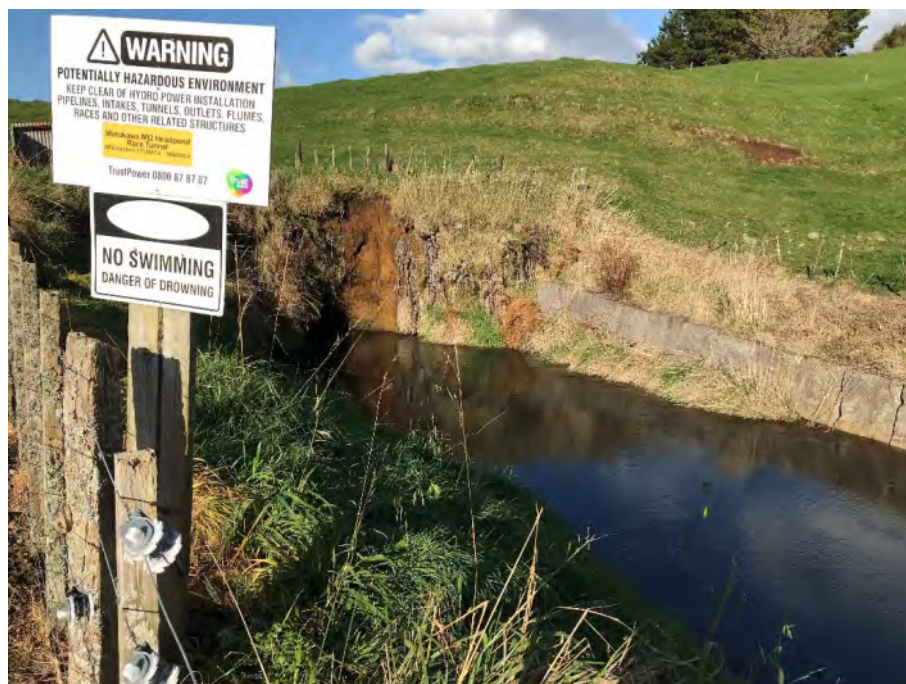
Photograph 8: Tunnel 1 Entrance. Note the low velocities and recent instability downstream of the mass concrete blocks.
