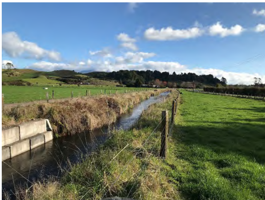
Photograph 5: View from CH 1225 upstream (June 2020). Note the low velocities and the mass concrete block repair.
