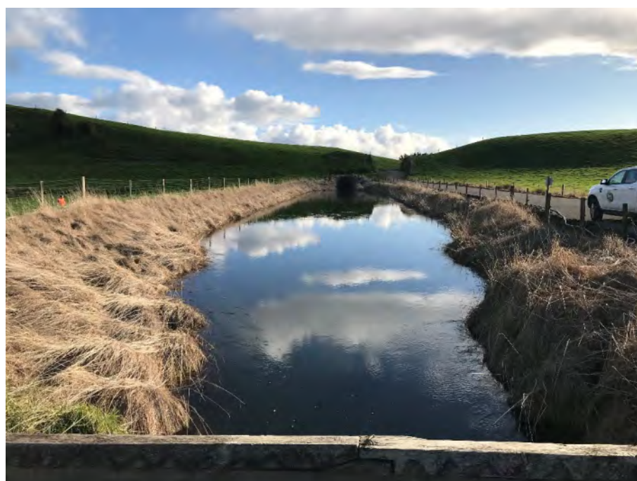
Photograph 9: View upstream from In-Race Generator. Note the low velocities.
