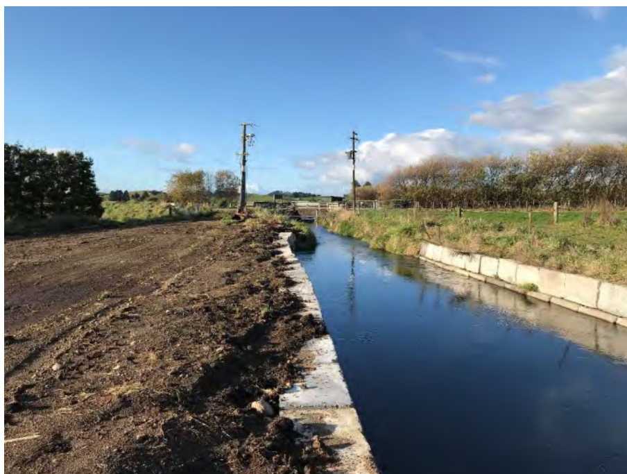
Photograph 12: Recent mass concrete block remedial works (June 2020). Note the relatively low velocities within the Race.
