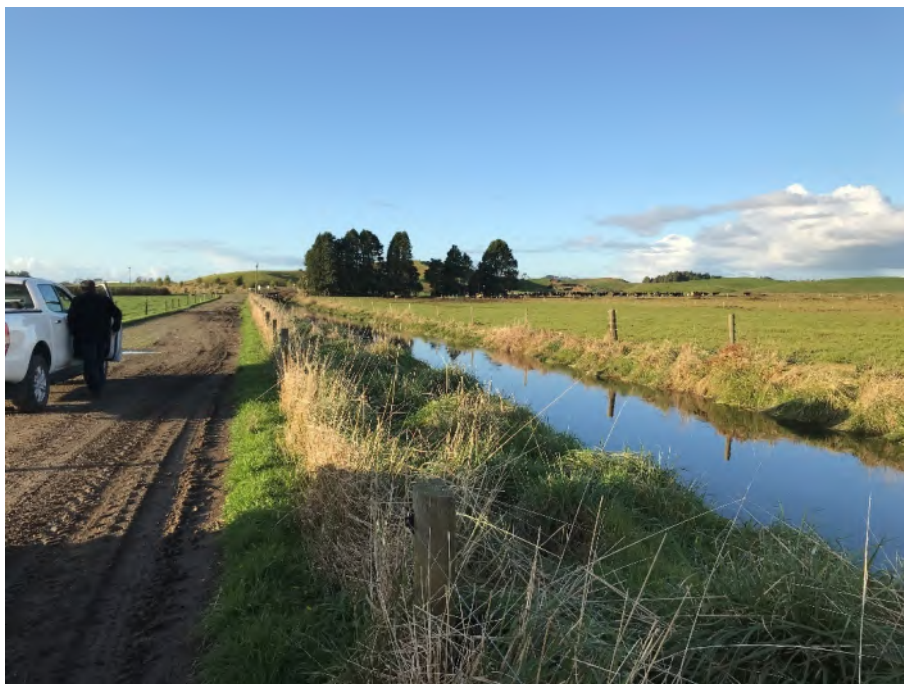
Photo 6: View downstream from CH 3400m (June 2020). The Race freeboard at the time of the inspection was estimated to be as low as 600mm on the true right bank. The ground levels in the paddocks beyond the right bank rise slowly. The true left bank (farm track) is significantly higher.
