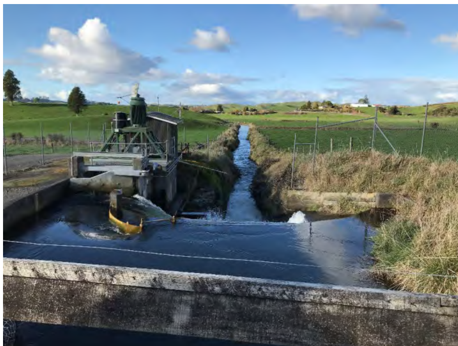
Photograph 10: View downstream from In-Race Generator (June 2020). Note the uneven appearance of the Race banks. The Upper Mangaotea Bridge is not visible (located around a left-hand bend).
