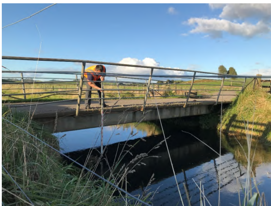
Photo 7: Lower Mangaotea Bridge with freeboard of 700mm (June 2020, lake level RL 198.4m).
