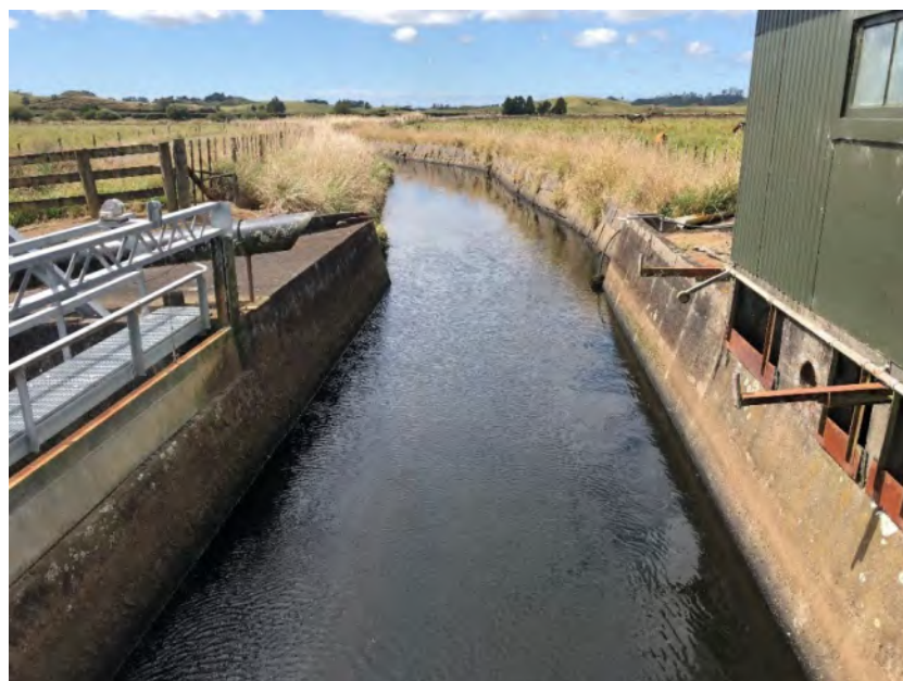
Photograph 14: View downstream from Mangaotea Aqueduct. Aqueduct is a concrete structure. Mass concrete blocks located on true right bank immediately downstream (February 2019 – low flows).
