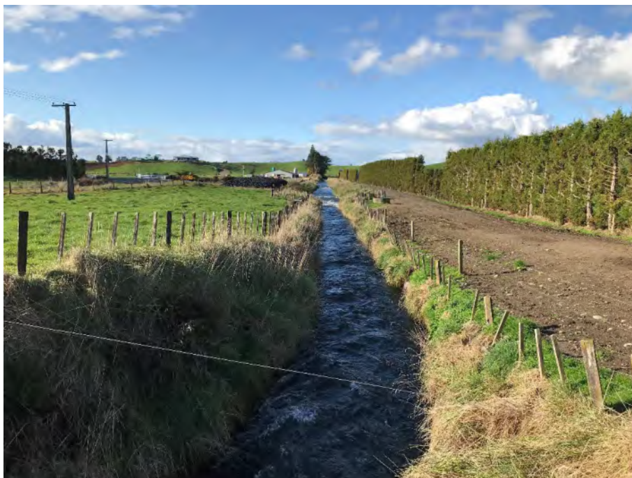
Photograph 7: View from Salisbury Road Culvert CH 1325 downstream (June 2020). Note the rapids further downstream (riprap lined).
