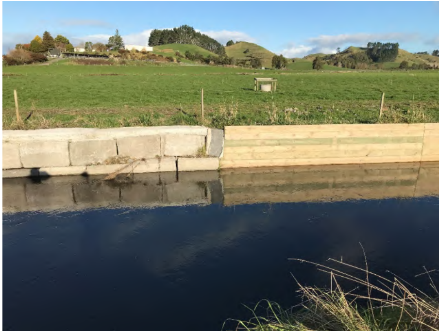
Photo 5: 900mm freeboard at CH 2660m on true left bank (June 2020). Note that the timber wall appears to extend above ground levels behind. Timber board are 150mm deep and the concrete blocks in the order of 600mm high.
