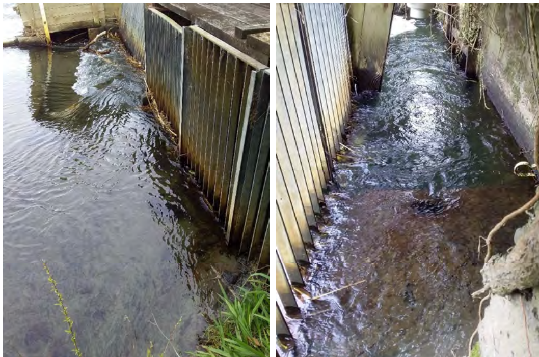
Photo 1 The intake screen in the Waiaua River at a high lake level (left) and behind the intake screen (right)
