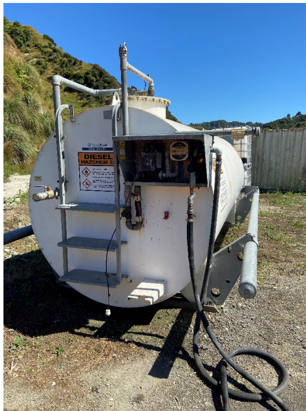
Photograph 6: Above Ground Diesel Storage Tank which will remain onsite
