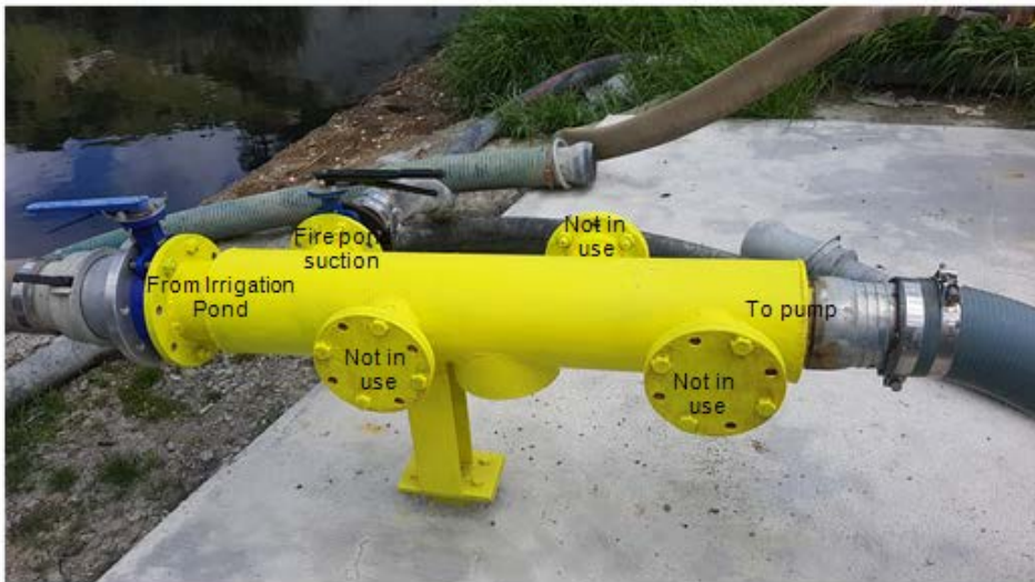
Pump Suction Manifold
