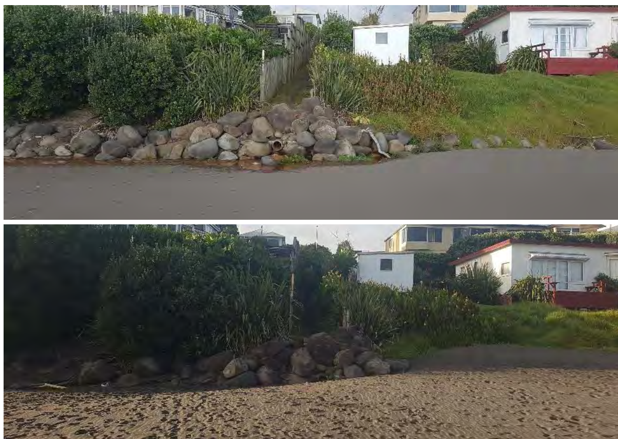
Photo 14 Messenger Terrace stormwater outlet at beach access (top: May 2019, bottom: April 2020)
