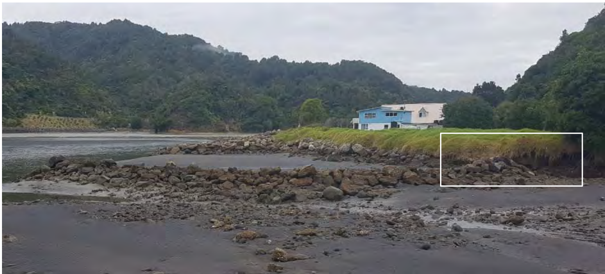
Photo 1 Tongaporutu rock groynes with section of scoured bank in white box, 1 May 2020
