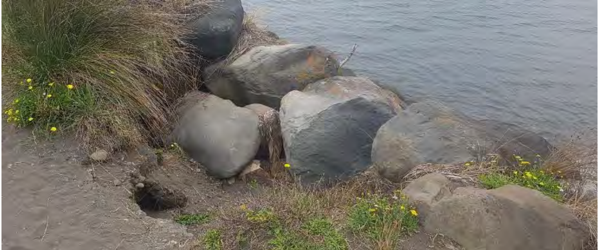
Photo 9 Small scoured section on Waiwhakaiho groyne, May 2020
