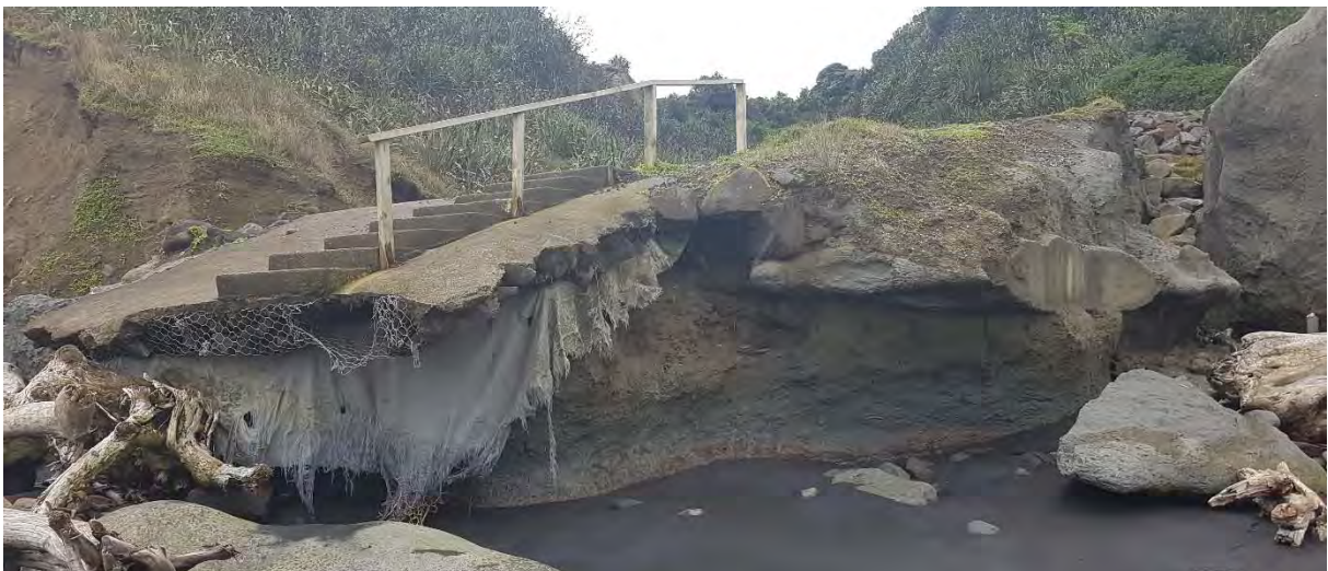
Photo 4 Remnants of Denby Road beach access structure consented under 6736 (April 2019)
