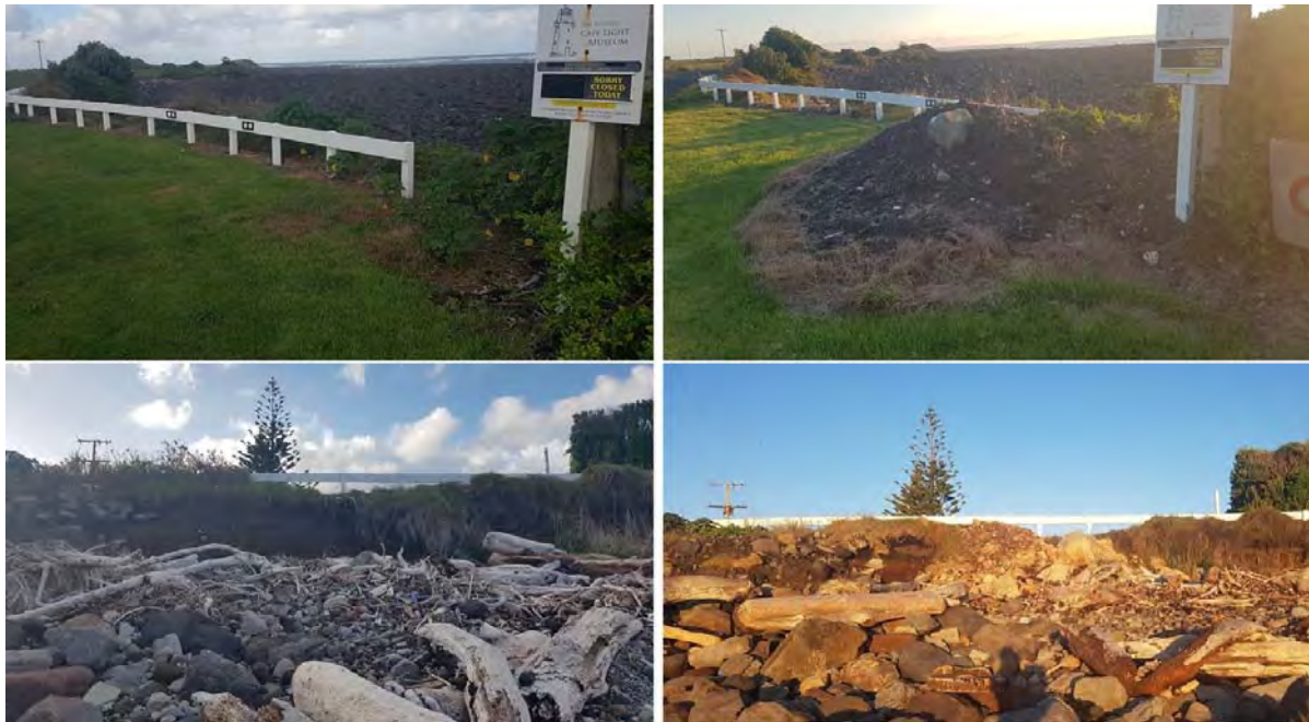
Photo 8 Bayly Road seawall before and after unauthorized works, 12 April 2019 (left), 6 May 2020 (right)
