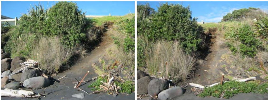
Photo 33 Close up of erosion present in front of Board Riders club caused by human foot traffic (June 2013 and May 2014)
