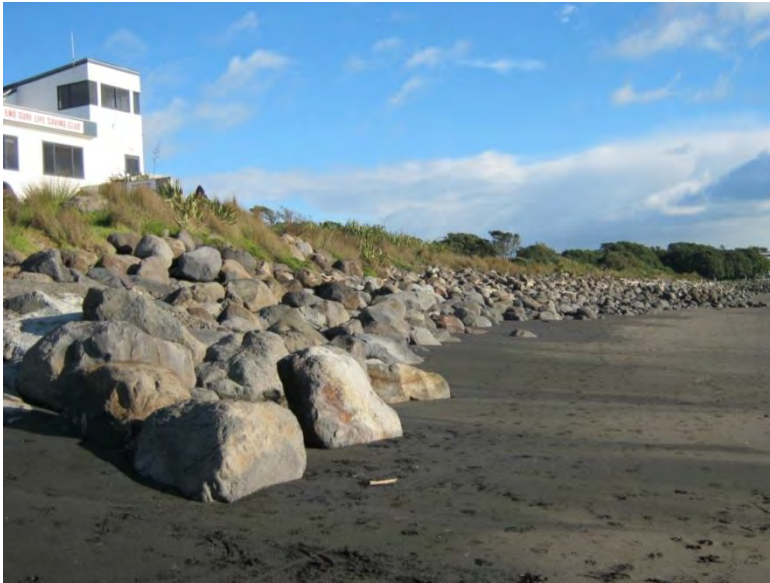
Photo 9 Rip rap seawall in front of East End Surf Life Saving Club (June 2013)
