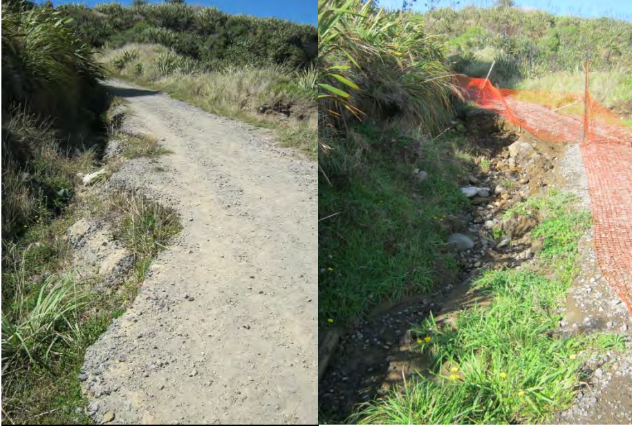
Photo 12 Erosion of beach track at the end of Denby Road left March 2013, right May 2014
