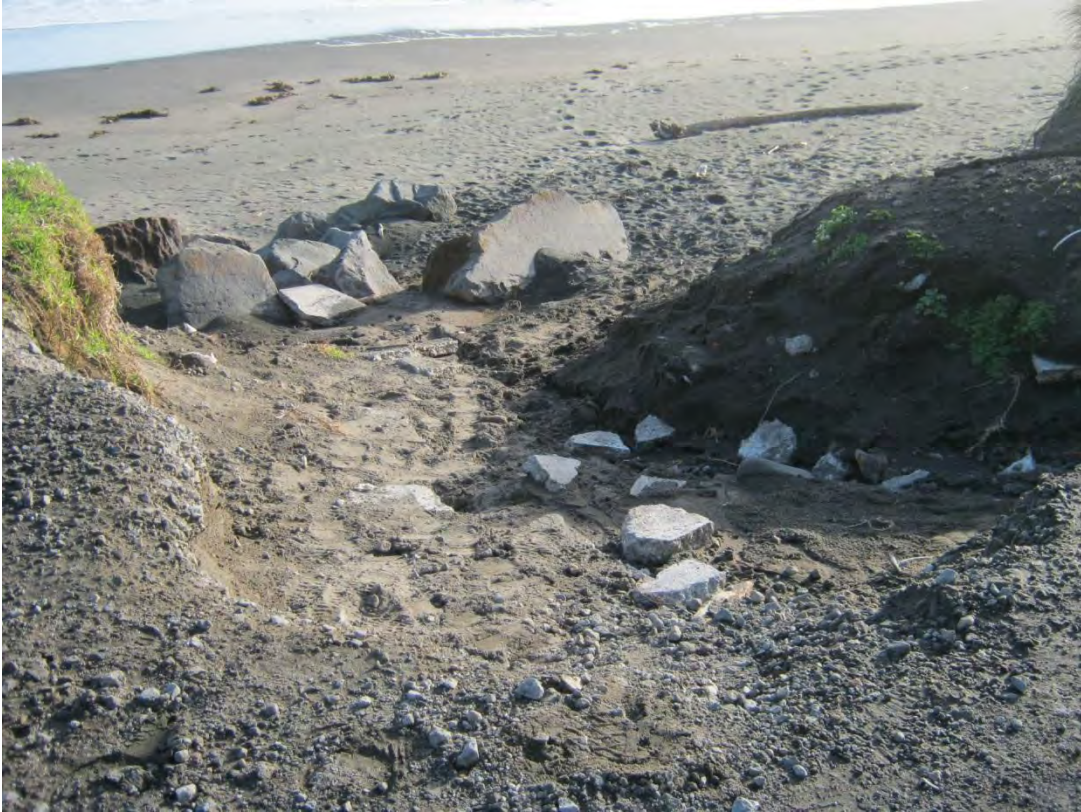
Photo 9 Erosion at the north-west end of the Middleton Bay seawall (May 2014)
