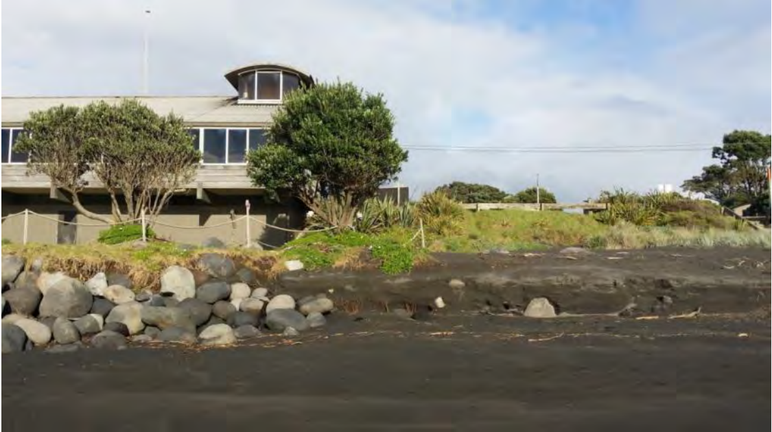
Photo 42 Protection works in front of Oakura Surf Lifesaving Club showing erosion of the bank/dunes to the west of the club (June 2015)
