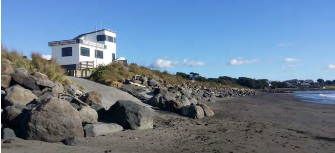
Photo 11 Rip rap seawall in front of East End Surf Life Saving Club (May 2015)
