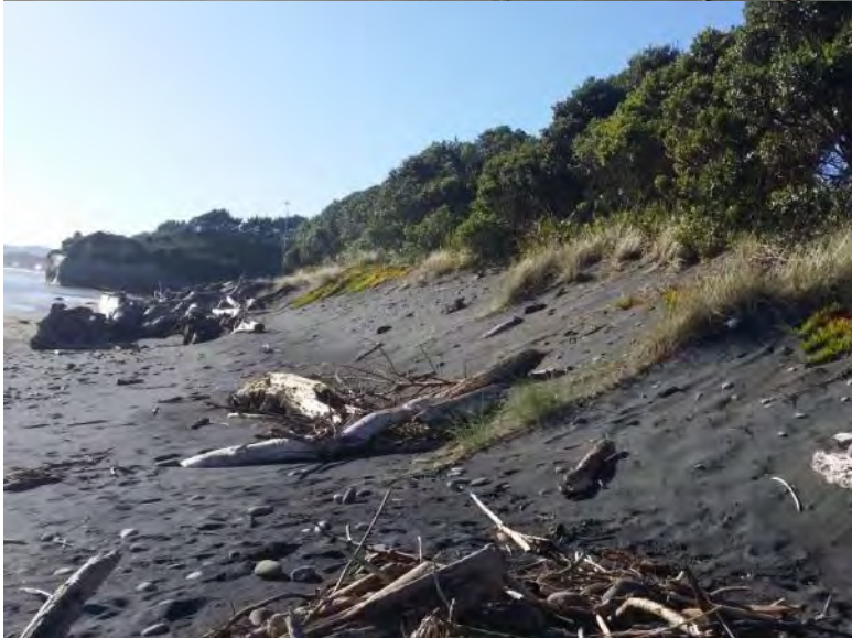
Photo 21 Urenui Rip rap protection wall extension (top May 2011, middle June 2013, bottom May 2015)
