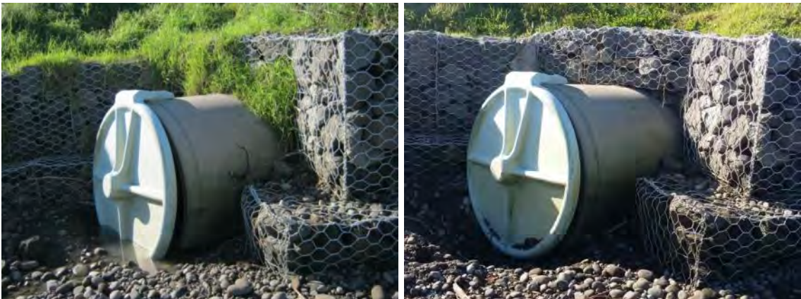
Photo 25 The stormwater outlet by the Atkinson Street/East Quay intersection (June 2013 and May 2015)
