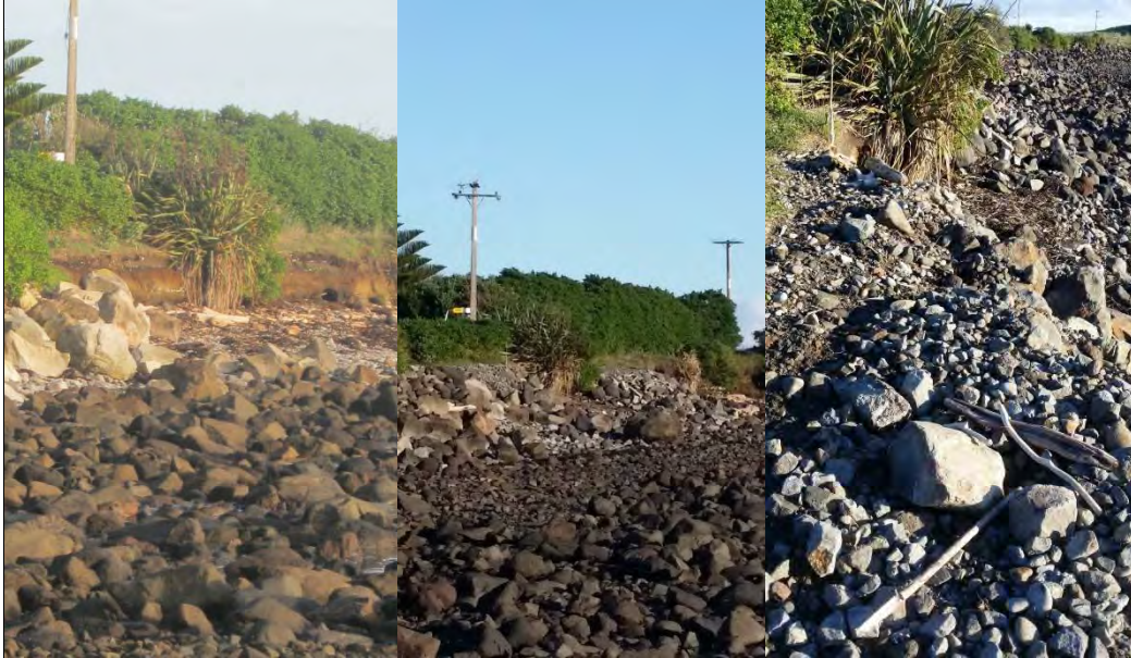
Photo 8 Left, erosion on the south side of the Bayly Road seawall May 2014, centre and right rubble used to prevent further erosion May 2015
