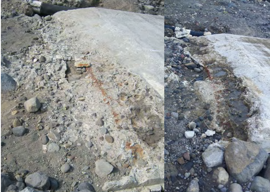
Photo 10 Top section of the Opunake Beach boat ramp (left March 2012, right May 2015)
