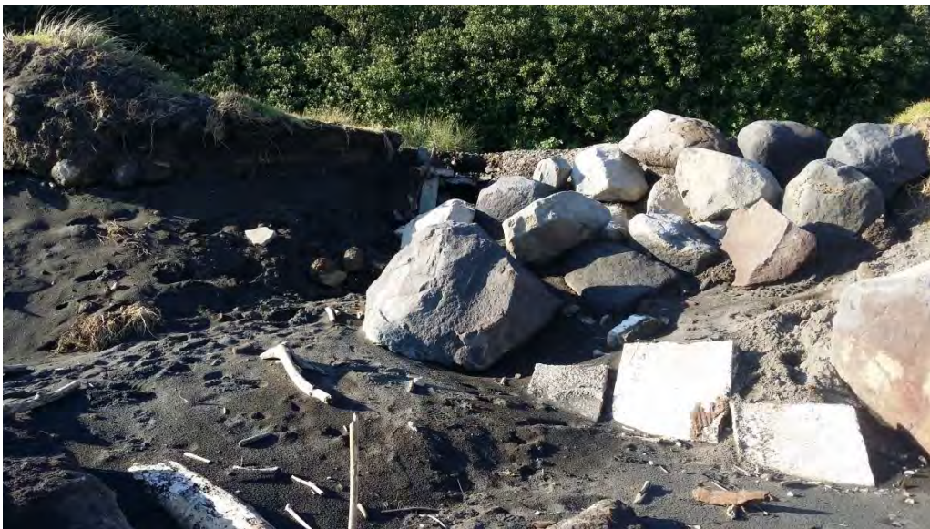
Photo 9 Erosion at the north-west end of the Middleton Bay seawall (May 2015)
