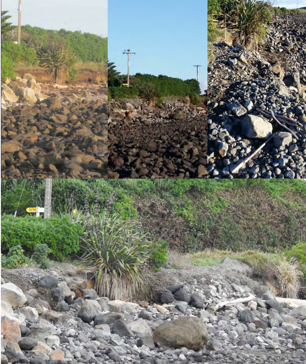
Photo 8 Bayly Road seawall (top left erosion on the south side of the seawall May 2014, top centre and right rubble used to prevent further erosion May 2015, bottom rubble remaining in place May 2016)
