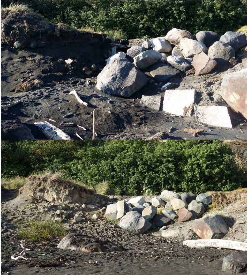
Photo 9 Erosion at the north-west end of the Middleton Bay seawall (top May 2015, bottom May 2016)
