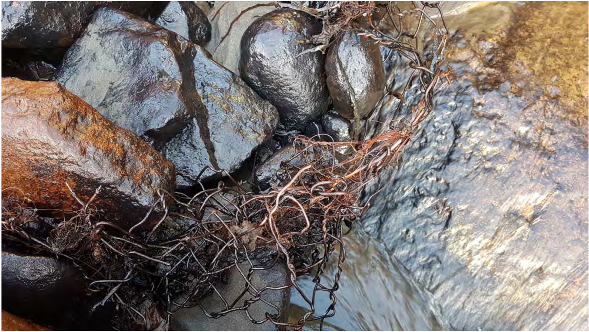
Photo 39 Outlet structure from the Hongihongi Stream showing to the left of the outlet were rusty and splitting gabion baskets (May 2017)
