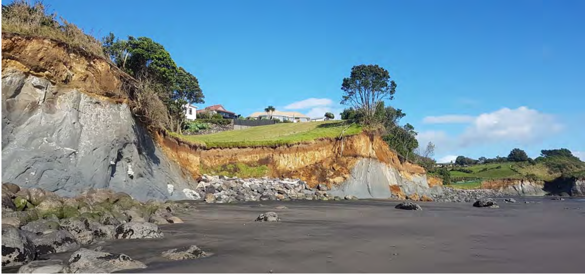
Photo 7 Eroding cliffs to the west of the seawall at Onaero (May 2017)
