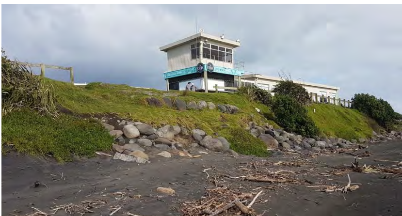
Photo 34 Rock protection works in front of Fitzroy Surf Lifesaving Club (top May 2015, middle June 2016, bottom May 2017)
