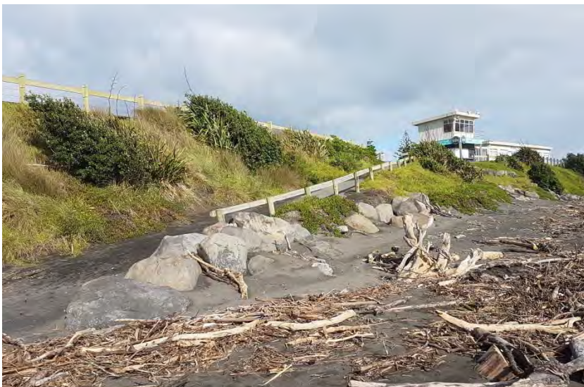
Photo 33 Boat ramp and rock protection works in front of Fitzroy Surf Lifesaving Club (top May 2015, middle June 2016, bottom May 2017)
