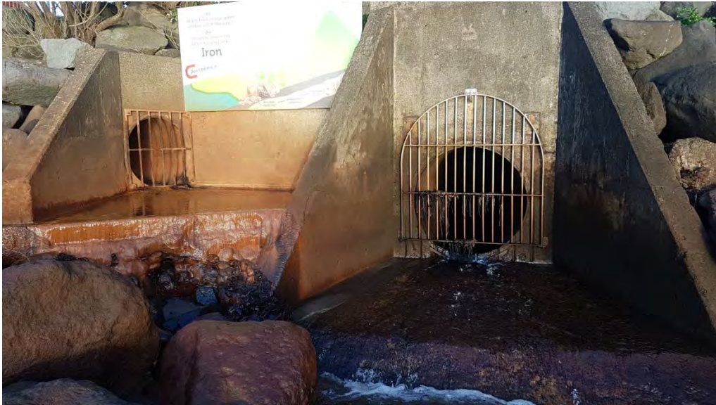
Photo 15 Hongihongi Stream outlet structure (May 2017)
