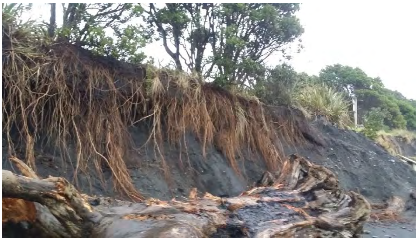
Photo 43 Erosion at the west end of Urenui Beach June 2016
