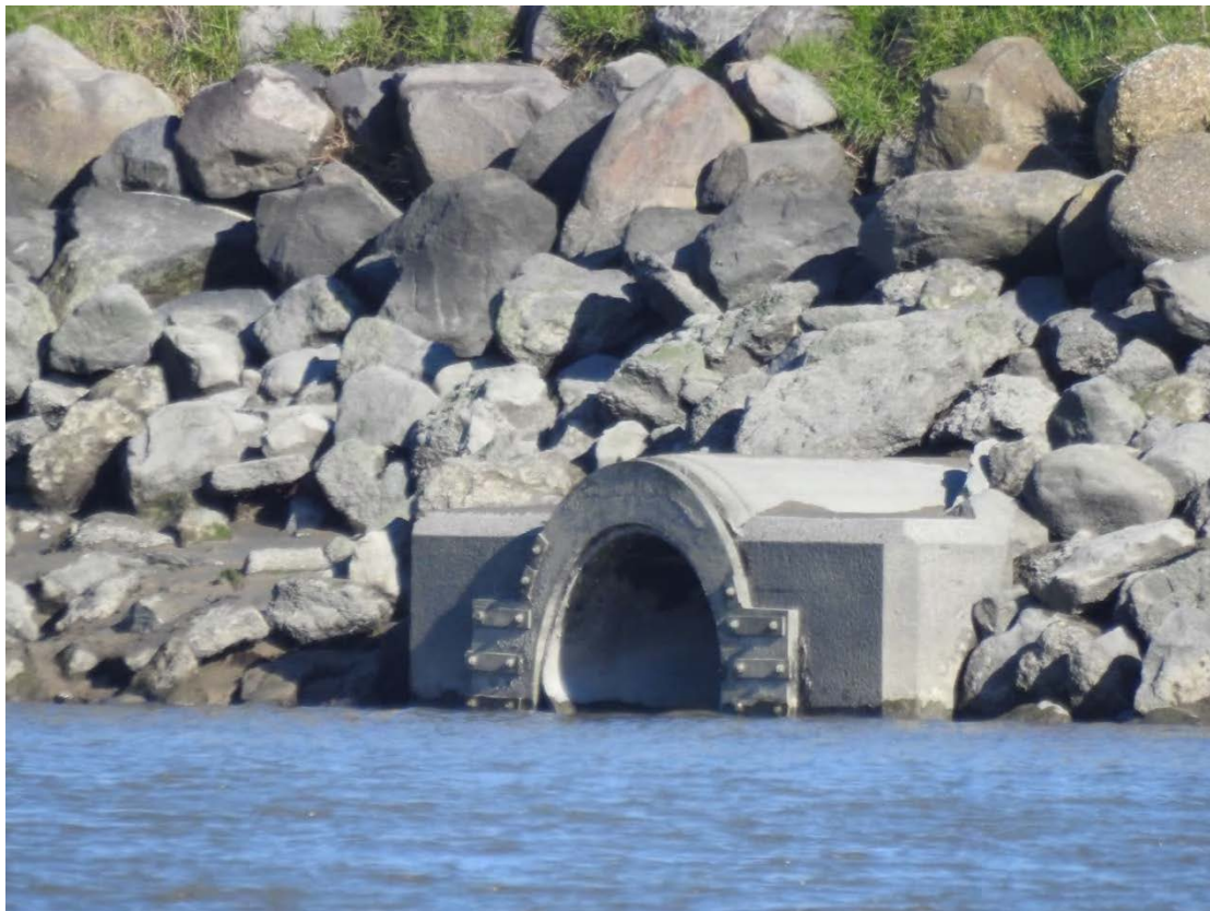
Photo 14 Stormwater outlet structure McNaughton Street, Waitara (June 2016)
