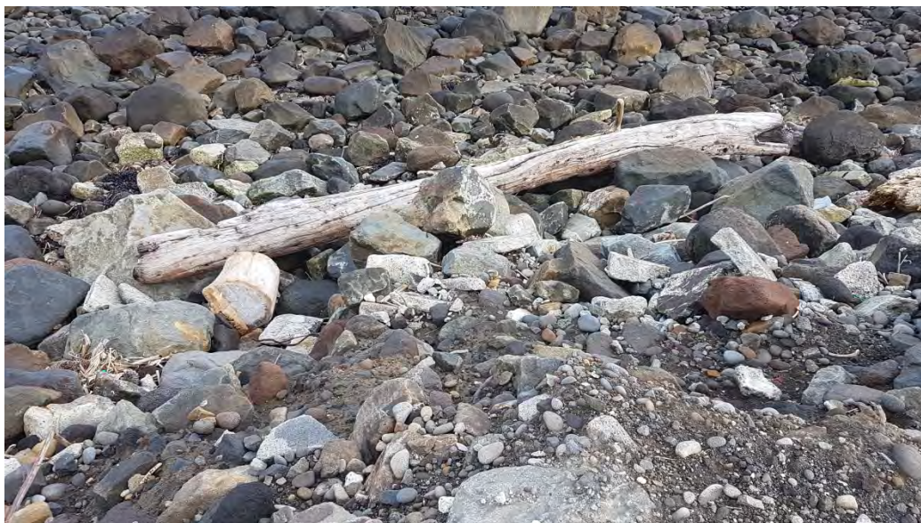
Photo 8 Bayly Road seawall (top rubble used to prevent further erosion May 2016, bottom rubble remaining in place April 2017)
