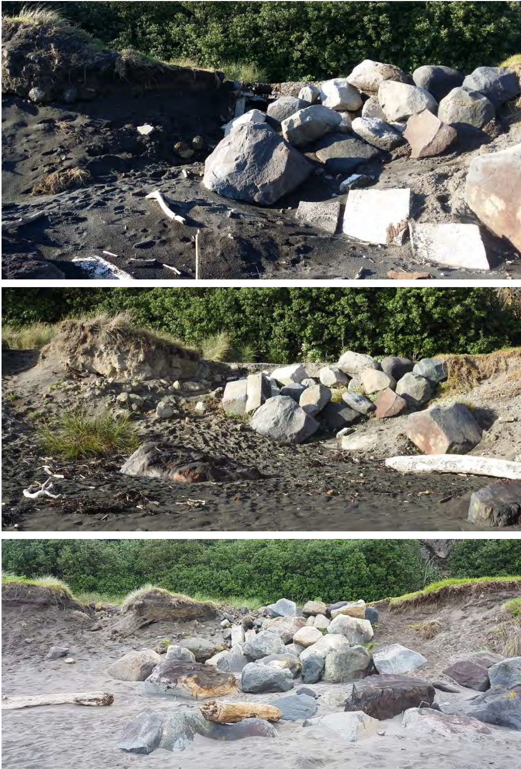
Photo 9 Erosion at the north-west end of the Middleton Bay seawall (top May 2015, middle May 2016, bottom April 2017)
