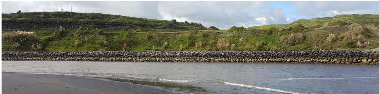
Photo 13 Training wall at Patea shown on the far side of the river (April 2017)
