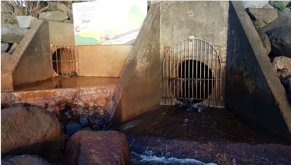
Photo 15 Hongihongi Stream outlet structure (May 2017)
