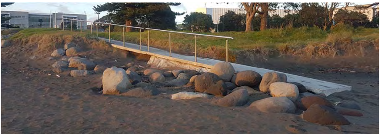
Photo 38 Damaged access structure at Ngamotu Beach (May 2018)
