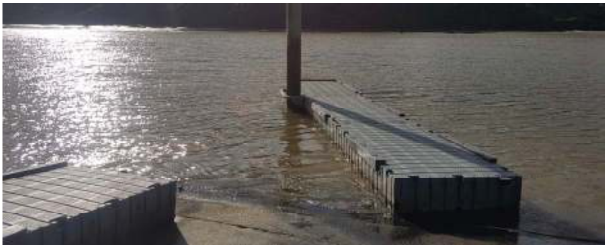
Photo 15 Damaged jetty at the Patea boat ramp, 22 May 2018
