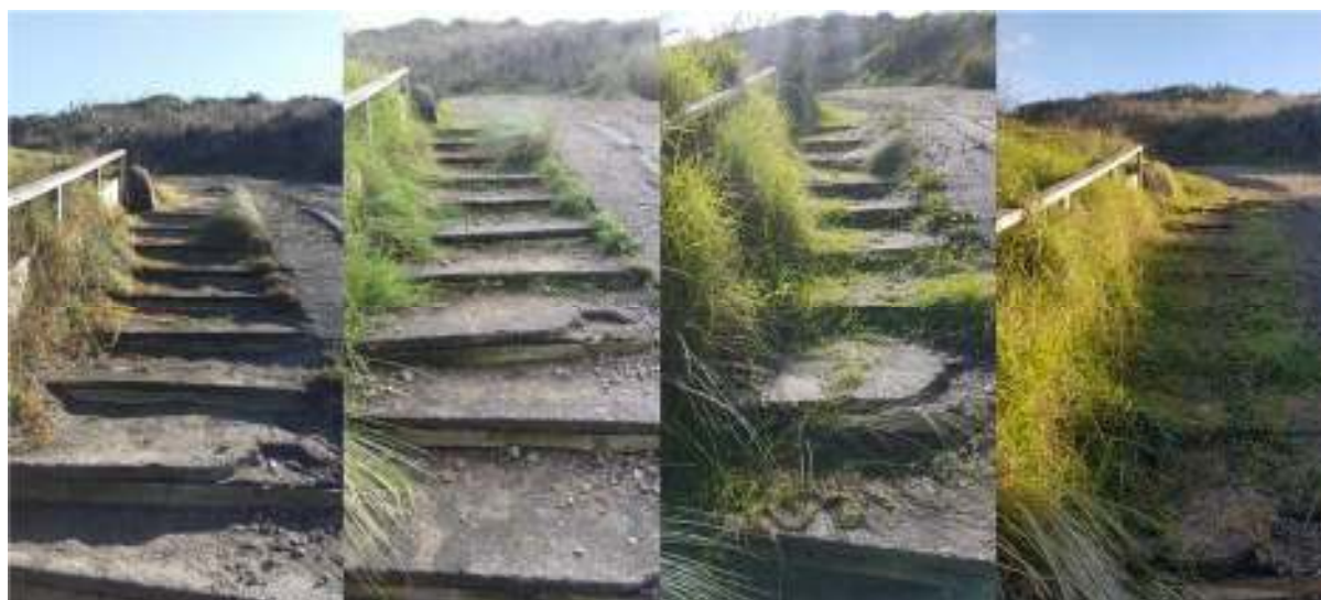
Photo 16 Deterioration of the Caves Beach access ramp (from left to right: May 2015, May 2016, April 2017 and May 2018)
