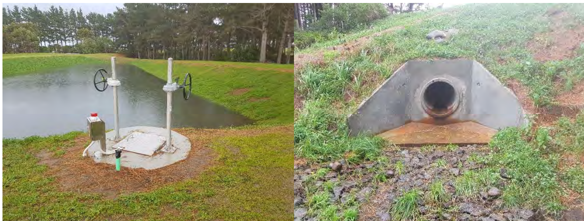
Photo 1 Northern stormwater pond, stop valves and outfall to the Kaupokonui Stream
