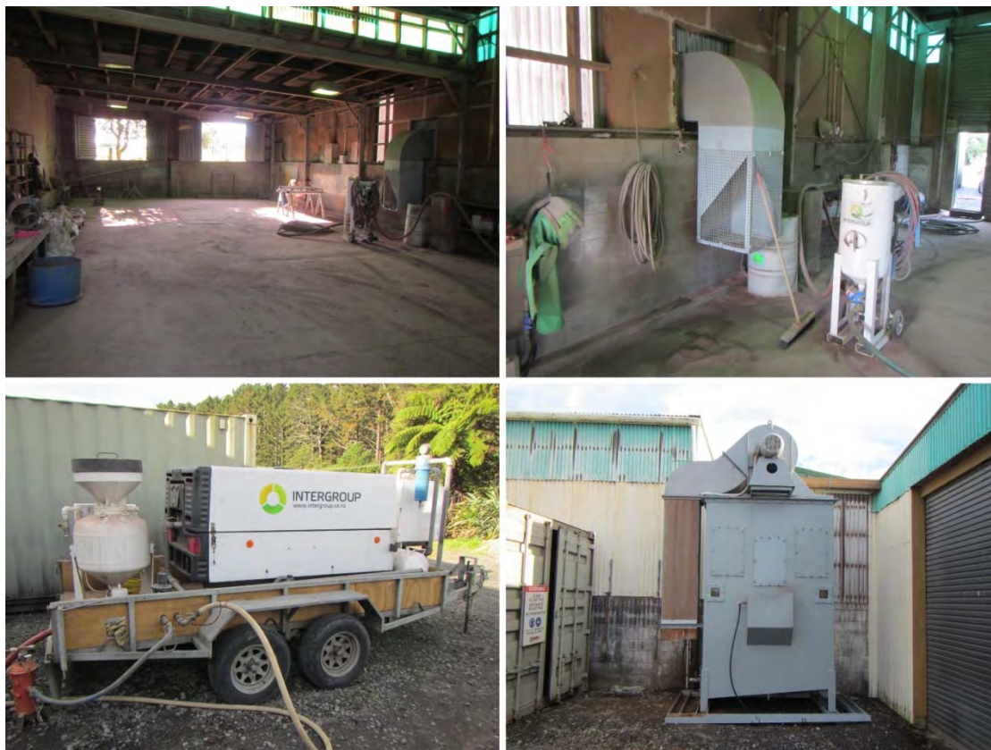
Photo 3 Site photos from Intergroup Ltd showing the blasting shed and key process equipment
