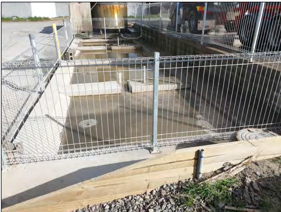
Photo 1 FBT's new truck wash treatment system.
