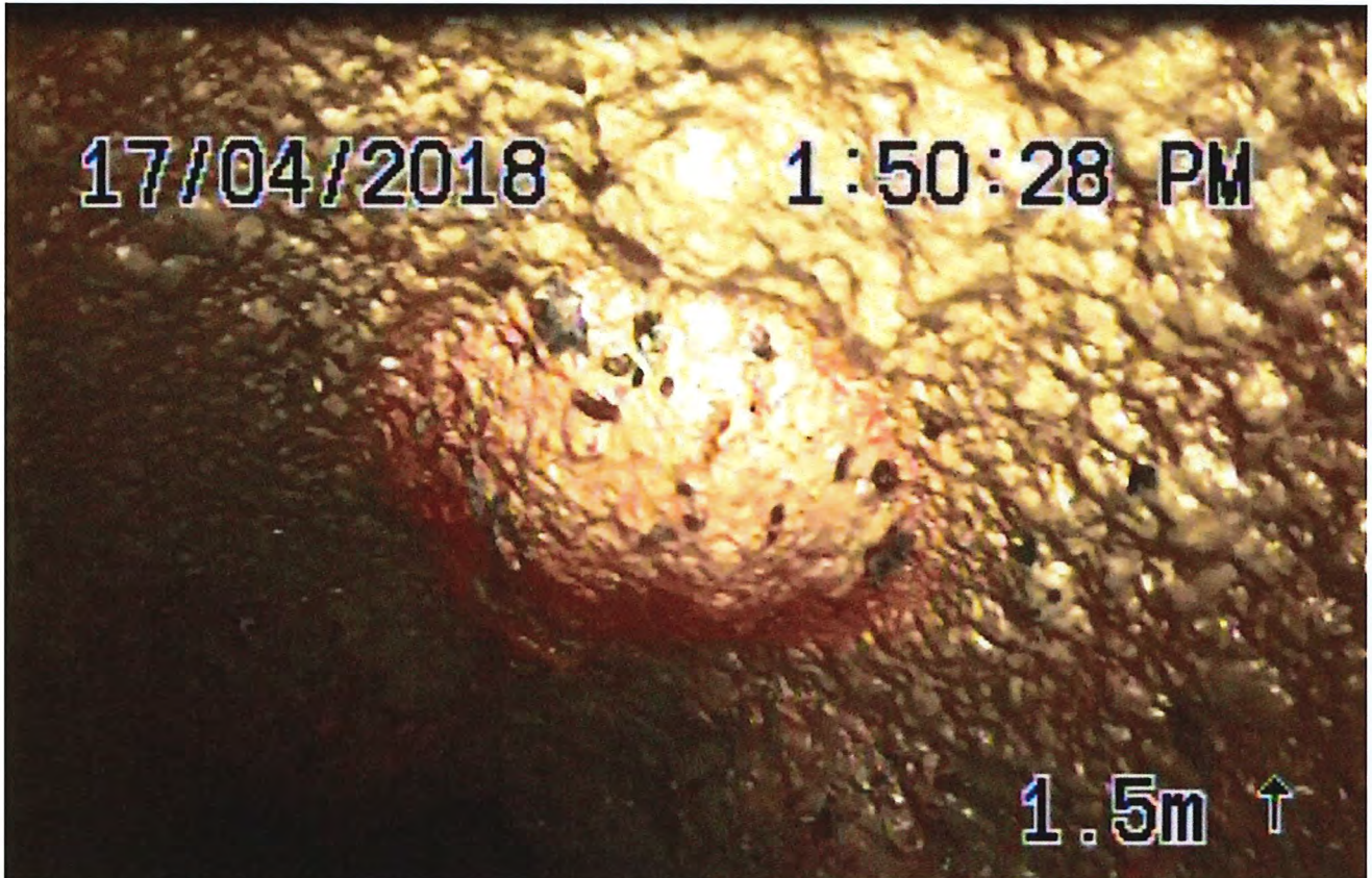
Solid growths in the riser pipe
