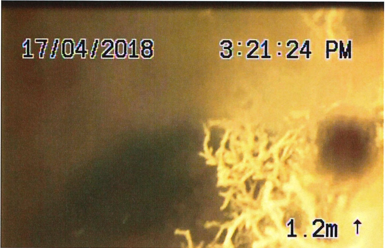
Organic material in the riser pipe.
