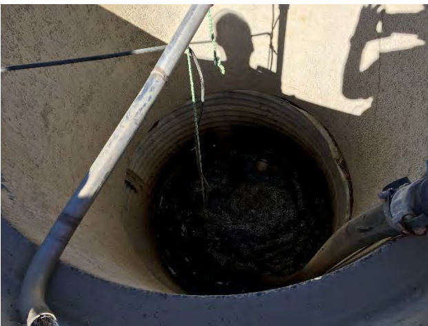
Figure 3: Leachate sump for TBE concentrated source biofilters showing large inlet flow.
