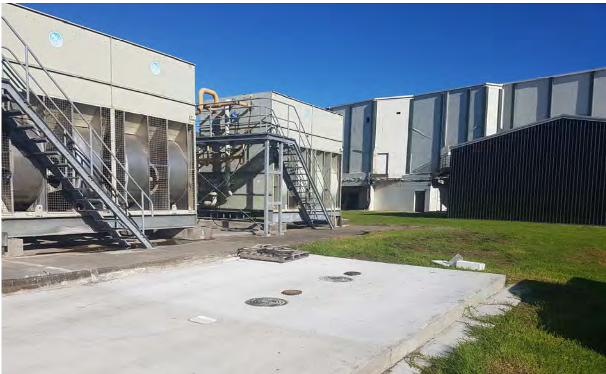
Photo 1 Dual stage smart chamber treatment system and underground sand filtration pit (19 May 2020)
