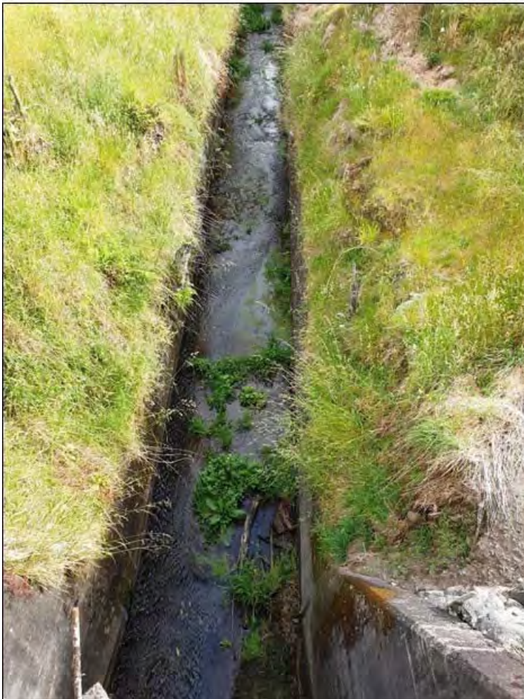
Photo 2 Old sluice gate leak (top) and race (bottom).
