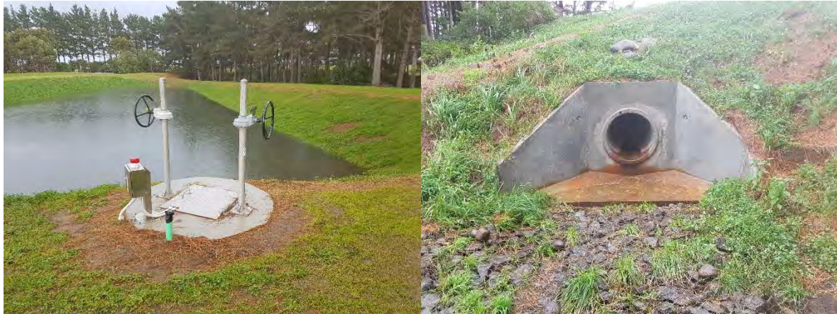
Photo 1 Northern stormwater pond, stop valves and outfall to the Kaipokonui Stream
