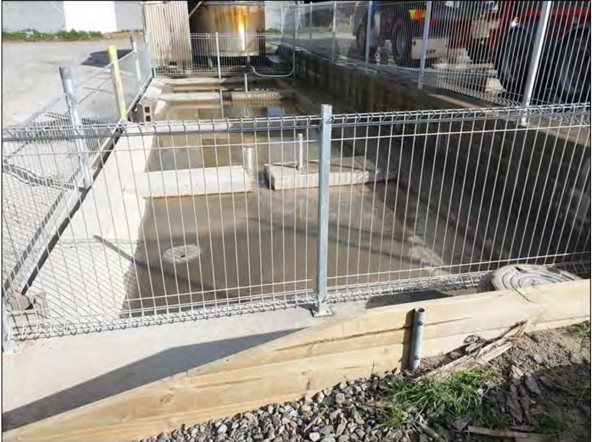
Photo 2 FBT's new truck wash treatment system.
