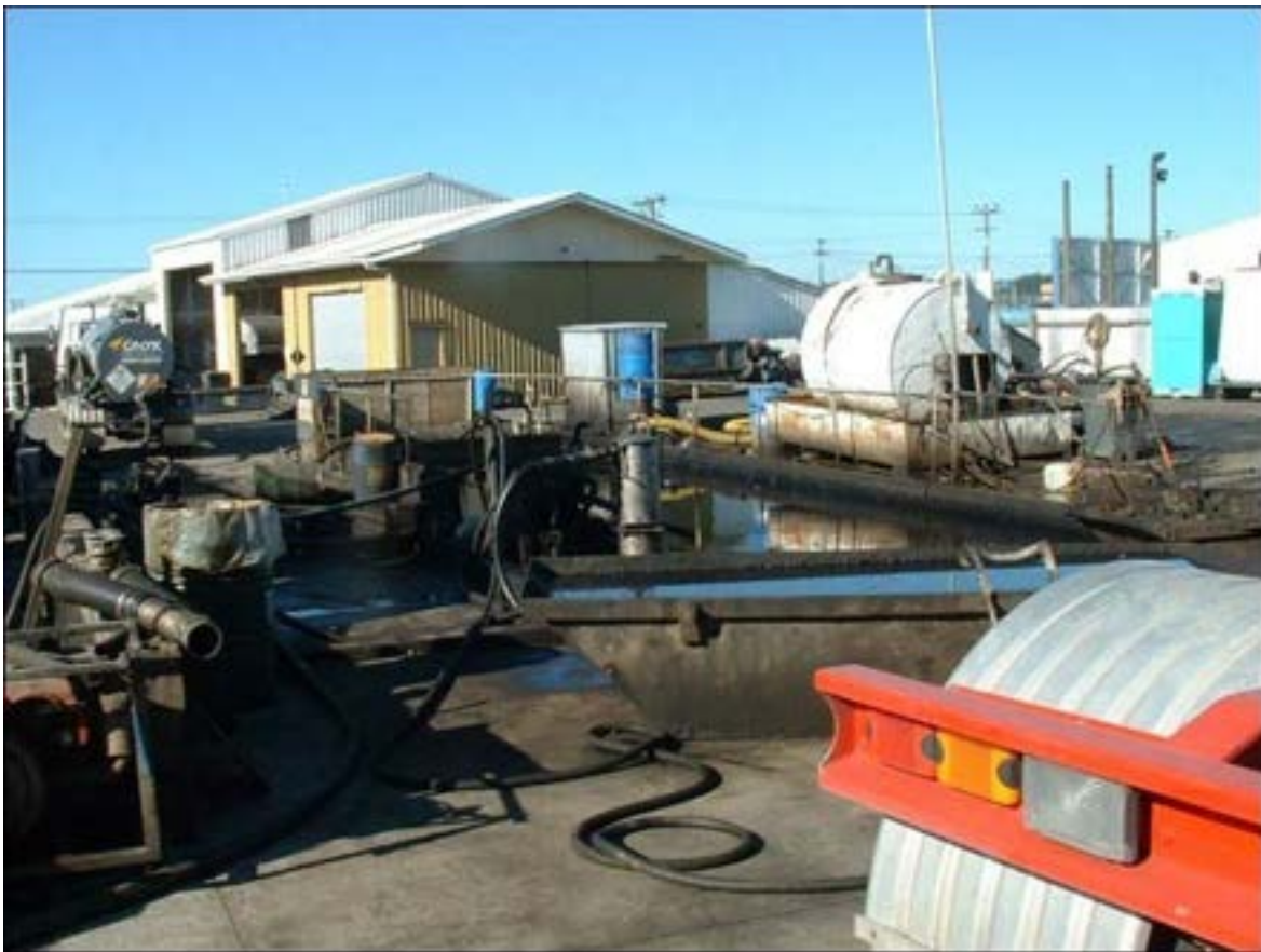
Photo 4 Intergroup Ltd oil treatment facility
