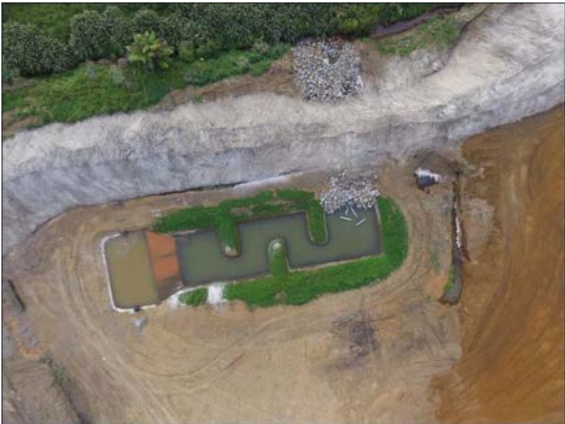
Figure 13 Aerial view of new sediment treatment pond at Taranaki Sawmills
