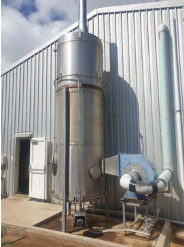
Photo 7 Zelum scrubber and associated bunding, September 2020
