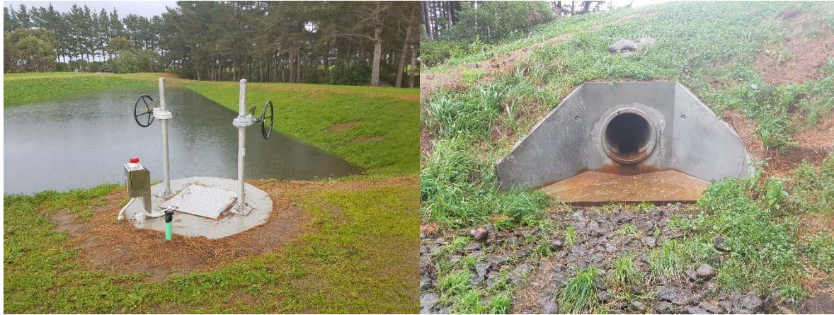
Photo 1 Northern stormwater pond, stop valves and outfall to the Kaipokonui Stream
