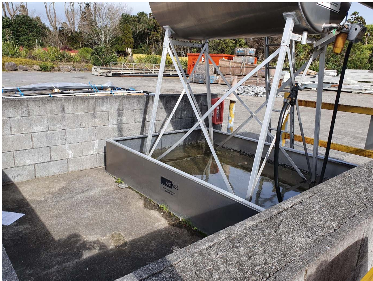
Photo 13 Hazardous chemical storage and bunding, July 2020
