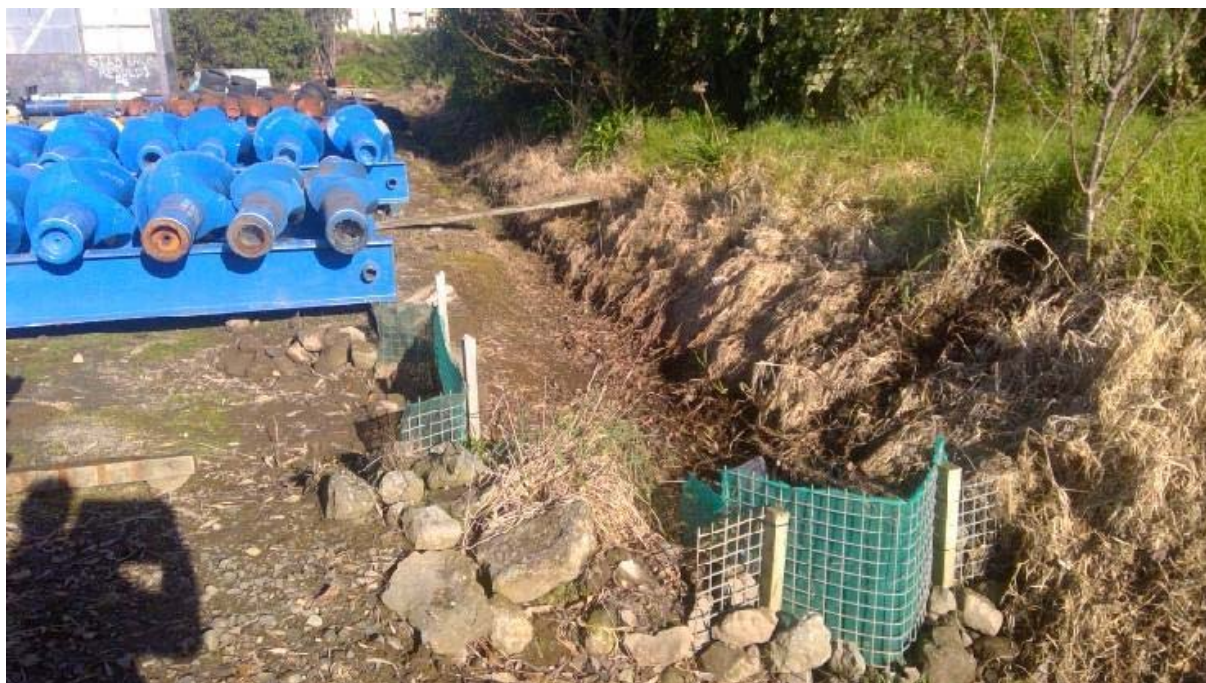
Photo 19 Sediment controls on Tasman Tools' perimeter drain, September 2020
