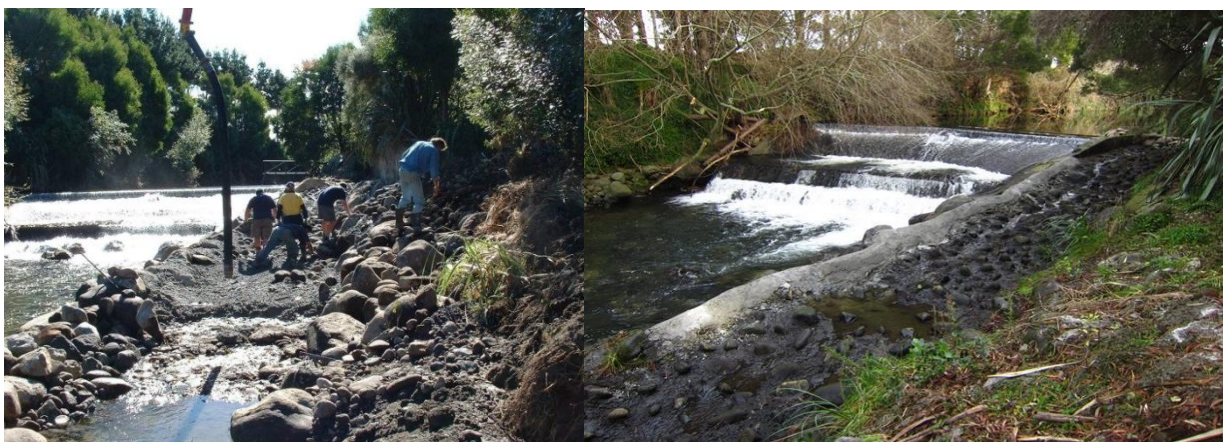
Photo 3 Construction of the new fish pass, March 2004, and repaired upper section, May 2013
