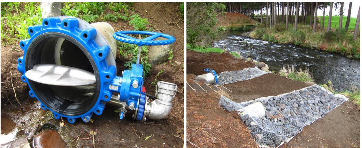
Photo 1 Valve on northern storm drain, 15 November 2012, and Reno mattresses laid out below storm drains to Kaupokonui River, 27 June 2013
