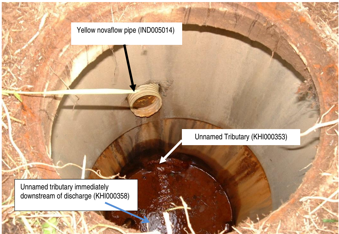
Photo 1 The view down manhole 1 including outlet of the unnamed tributary, the yellow novaflow pipe from the Taranaki Galvanizers site (IND005014) and the tributary immediately downstream of the discharge (KHI000358)
