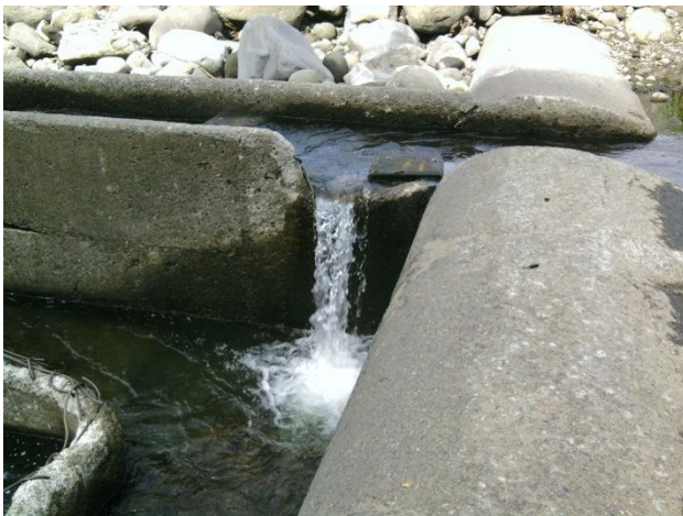
Photo 1 Small breakage in wall of fish pass, August 2012
