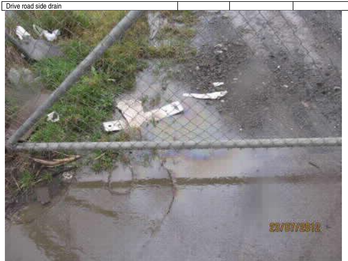
Photo 9 Visible sheen, overland flow from Meredith Scrap Metals Ltd 23 July 2014
