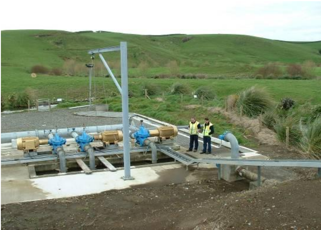
Photograph 2 Tawhiti water intake
