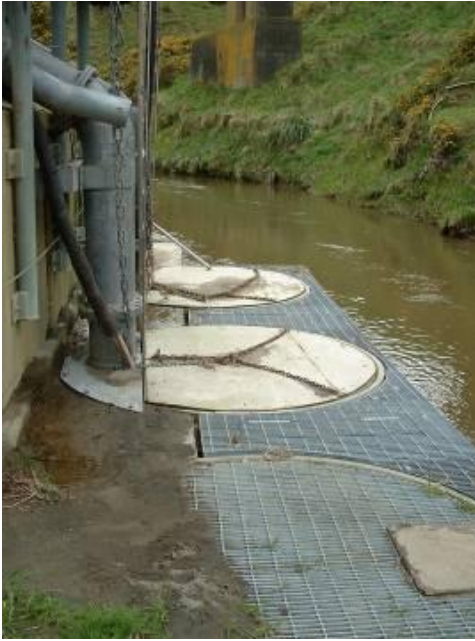
Photograph 5 Tangahoe River intake
