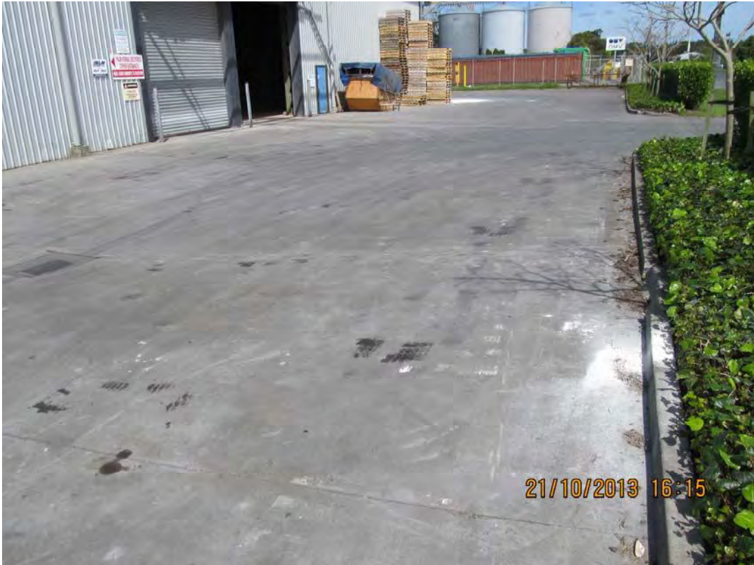
Photo 3 BLM Feeds – tracking from storage shed, 21 October 2013
