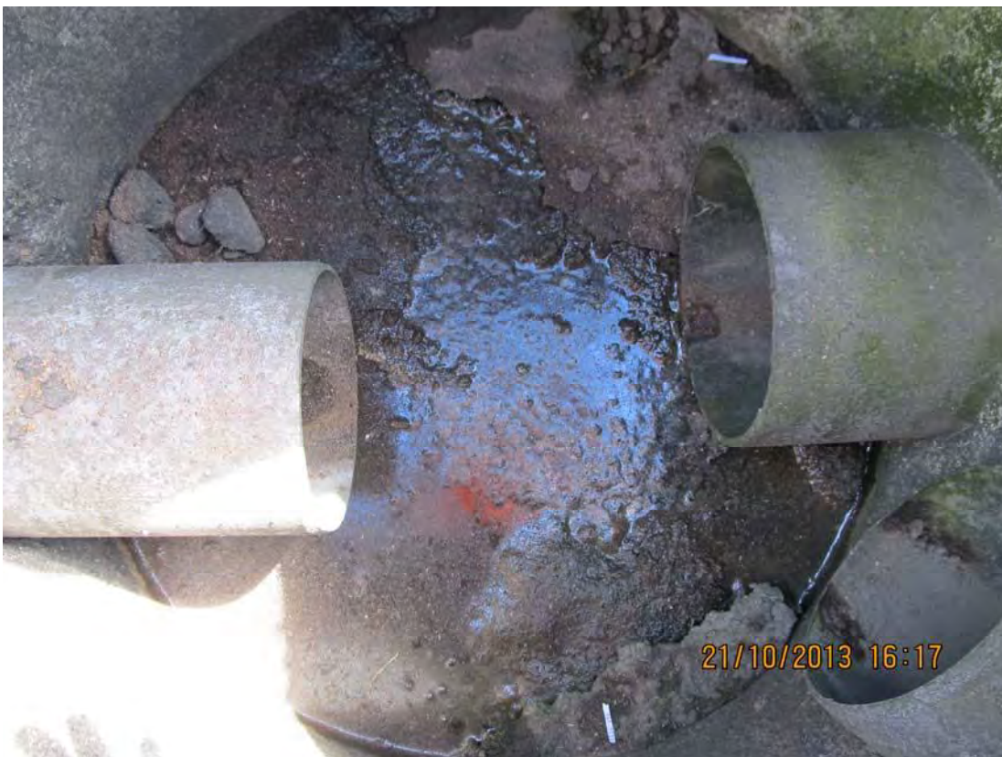
Photo 4 BLM Feeds – organic matter in stormwater sump, 21 October 2013
