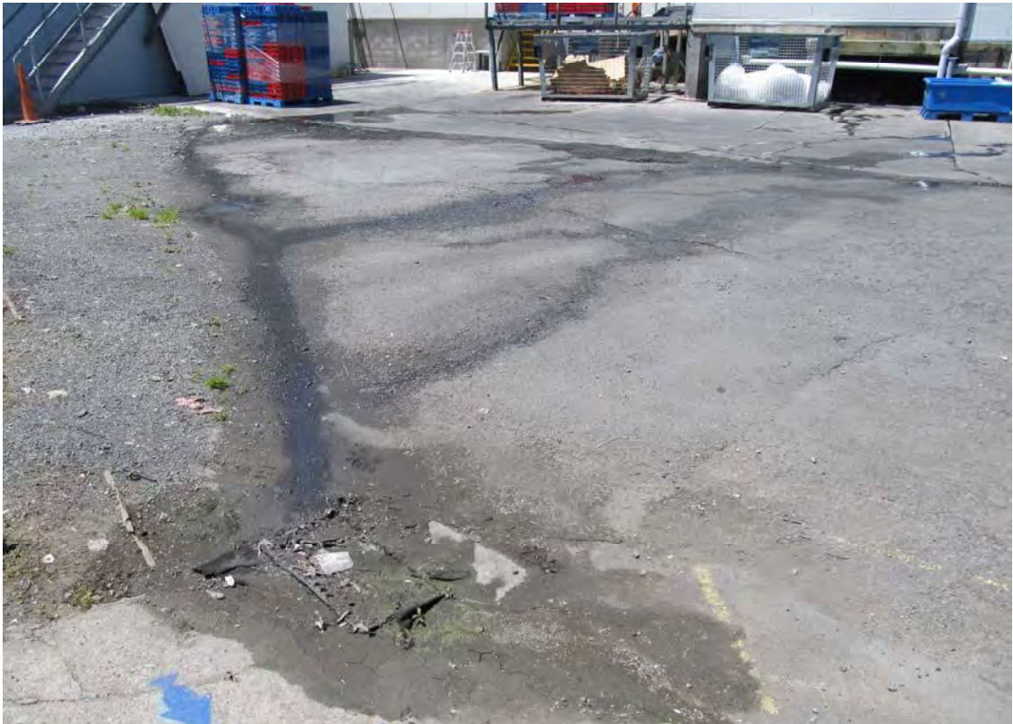
Photo 7 Tegel poultry processing plant leak from free flow building, 2 December 2013
