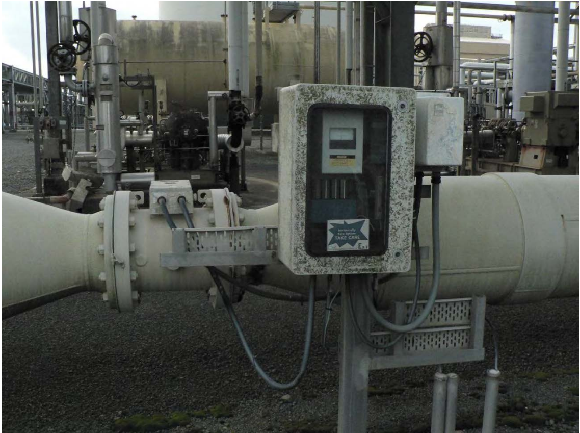
Photo 2 Motunui Raw water flow meter
