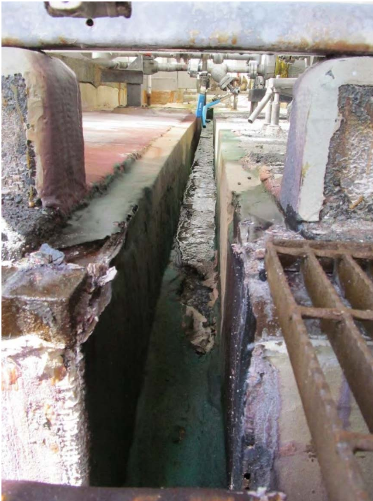
Photo 4 Point of discharge – the hole in the concrete channel
