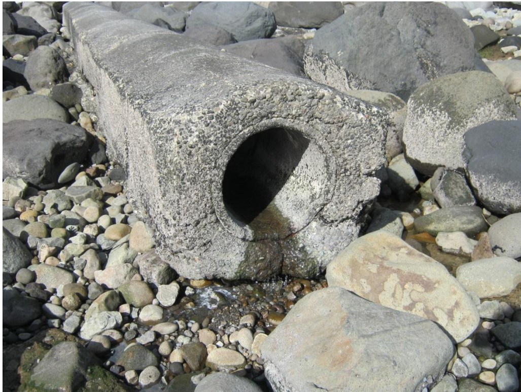
Photograph 1 Todd Energy Aquatic Centre discharge pipe
