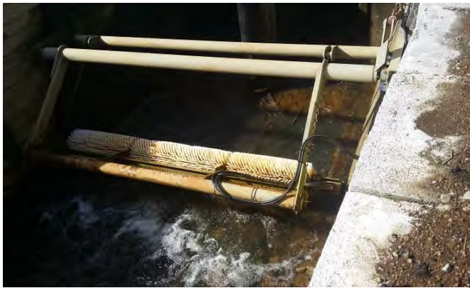
Photo 9 The Mangaotea Pumps intake and screen cleaning brush
