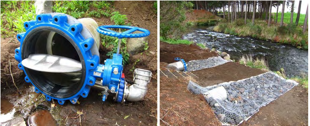
Photo 1 Valve on northern storm drain, and Reno mattresses laid out below storm drains to Kaupokonui Stream
