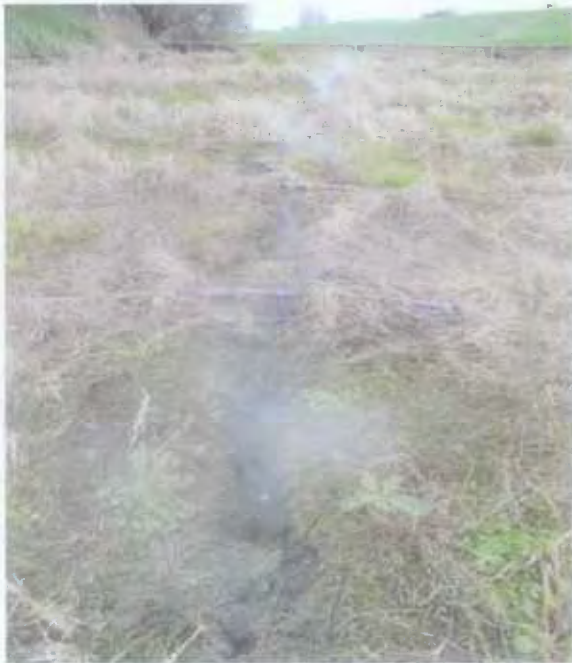
Figure 2: TBE concentrated, sources biofilter bed, with vapour leaking above one of the main ducts.
