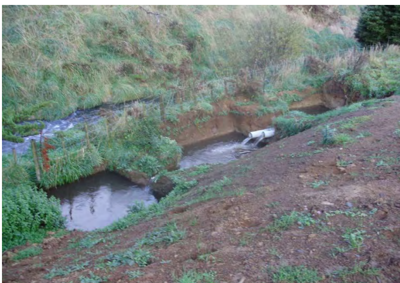
Photograph 2 The settling system at Taranaki Fish and Game trout hatchery
