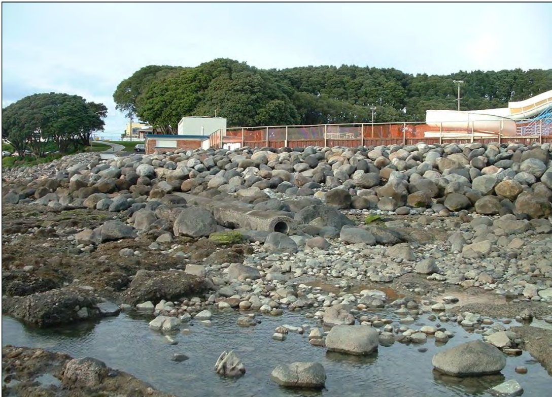
Photograph 1 Todd Energy Aquatic Centre ocean outfall
