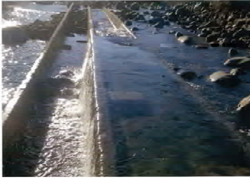
Photo 1 Fishpass debris accumulation after June 2015 floods
