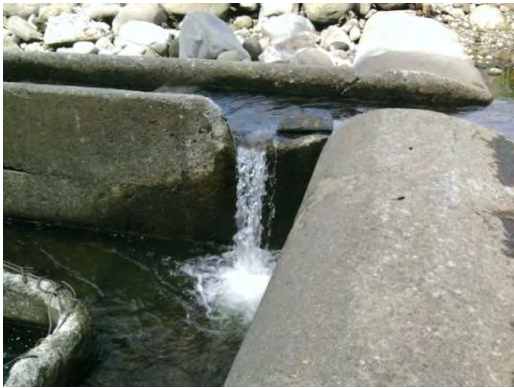
Photo 2 Breakage of wall of fish pass, August 2012
