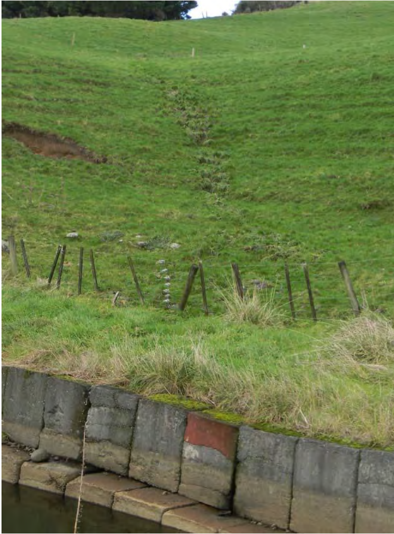
Photo 6 Evidence of recent surface runoff leading to the race just upstream of the in-race generator, 22 June 2015
