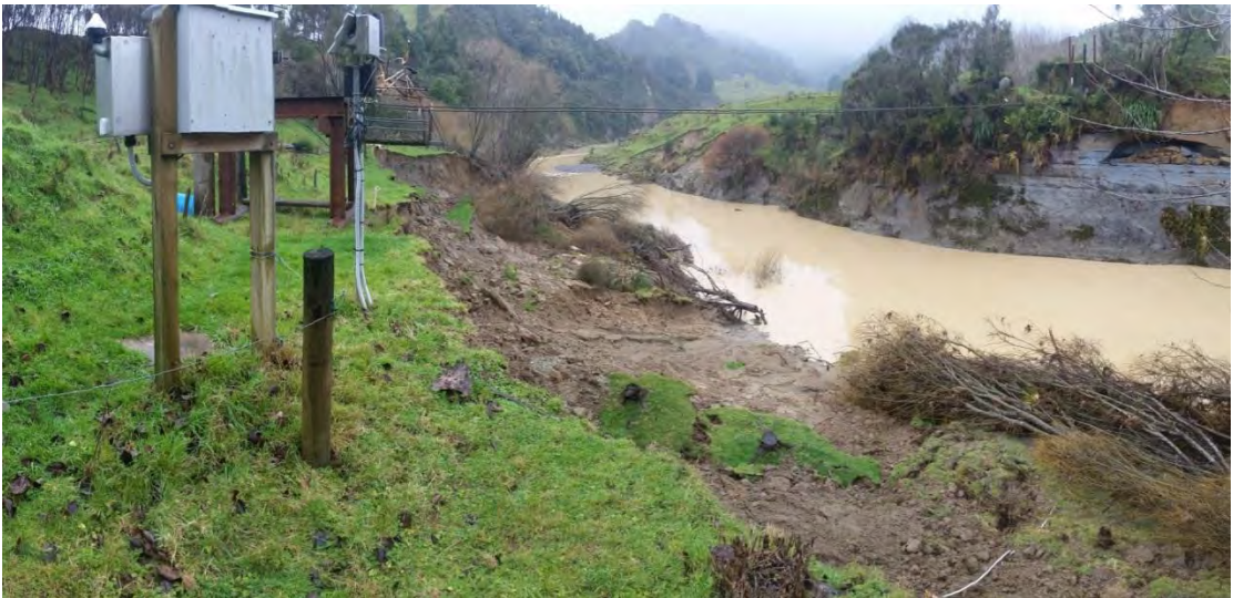
Photo 7 Bank slumping at the McColl's quarry recorder site, 7 July 2015.
