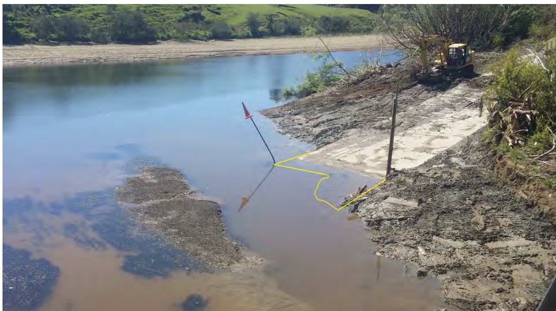
Photo 2 The Glen Nui boat ramp during a low lake level, 15 October 2015. The yellow line approximates the edge of the concrete ramp.
