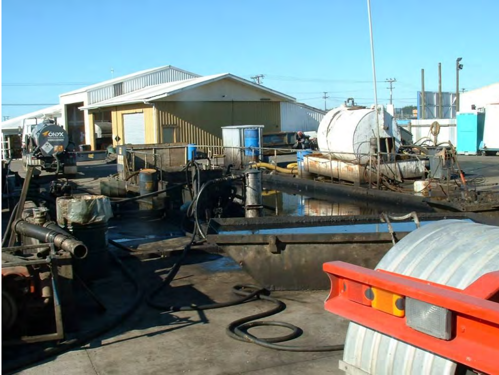
Photo 4 Intergroup Limited oil treatment facility
