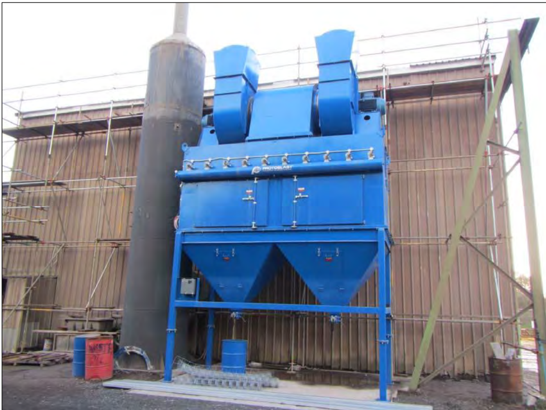
Photo 3 Newly installed Blastquip fabric filter air treatment system at Fitzroy Engineering
