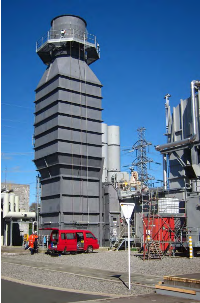
Photo 2 Stack testing at Stratford Peaker Plant GT21, 27 August 2014
