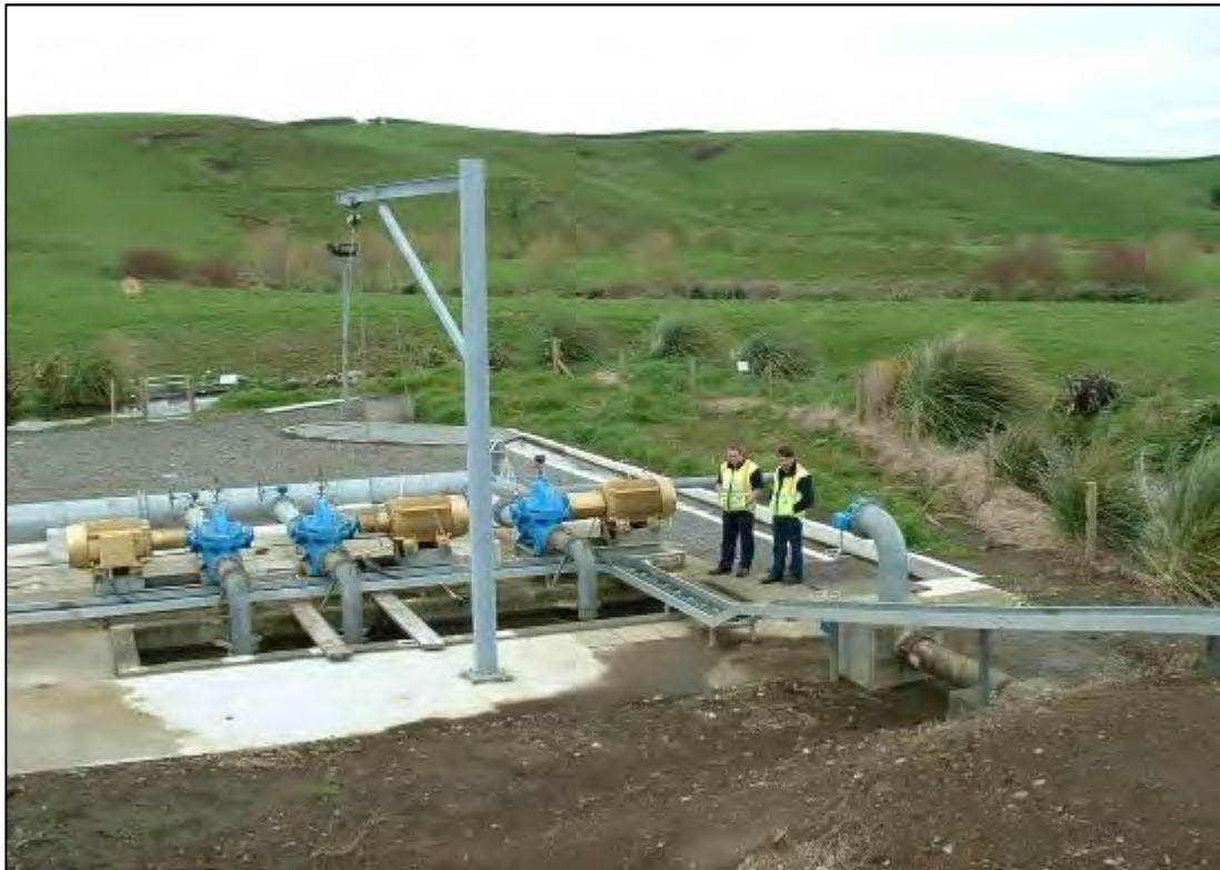
Photo 2 Tawhiti water intake
