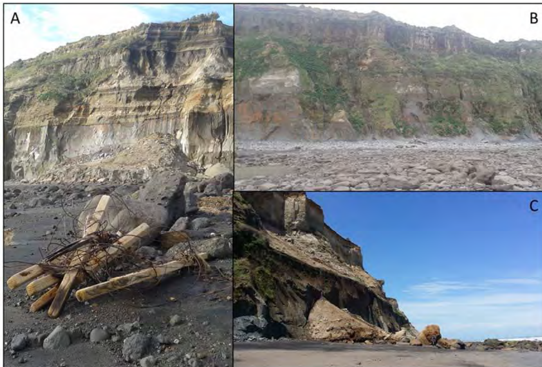
Photograph 9 Significant erosion over the reef site 200 m SE of the outfall October 2015 (A), Relatively intact cliffs covered in vegetation above the Pukeroa Reef site October 2015 (B), A large slip above Waihi Reef November 2015 (C)
