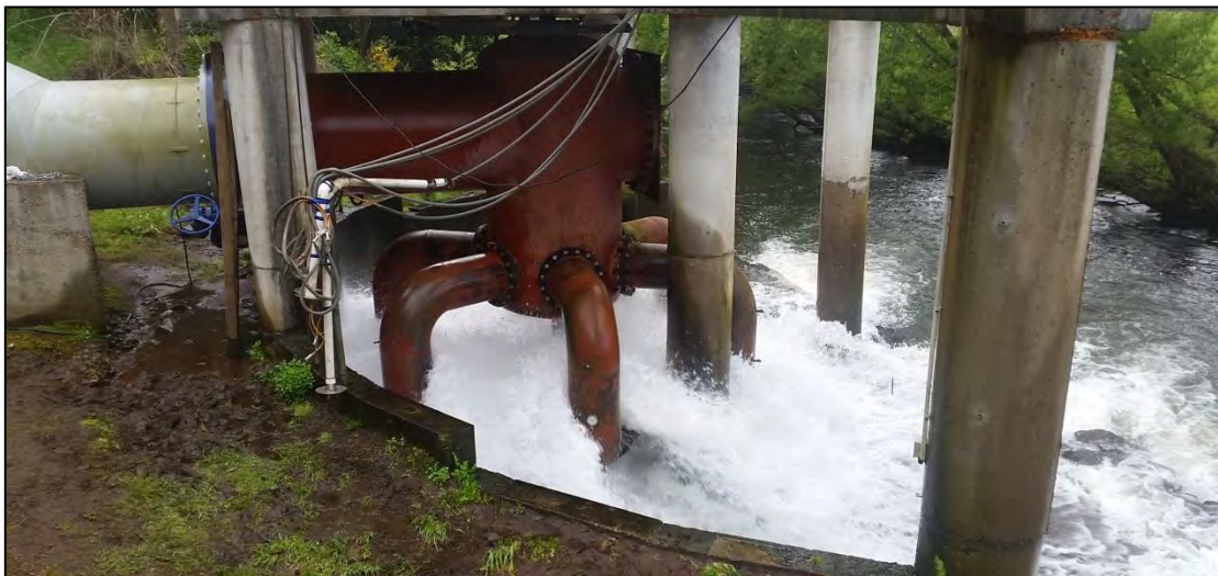
Photo 2 The station operating, 16 October 2015.
