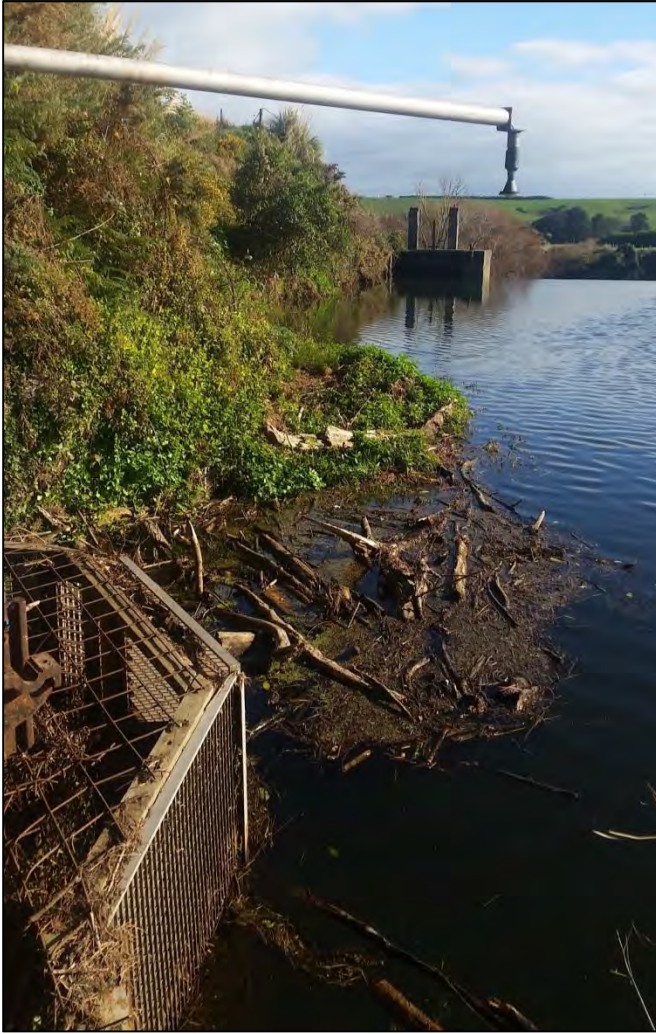
Photo 4 The intake and water level recorder (radar) positioned over the water where logs and other debris accumulates
