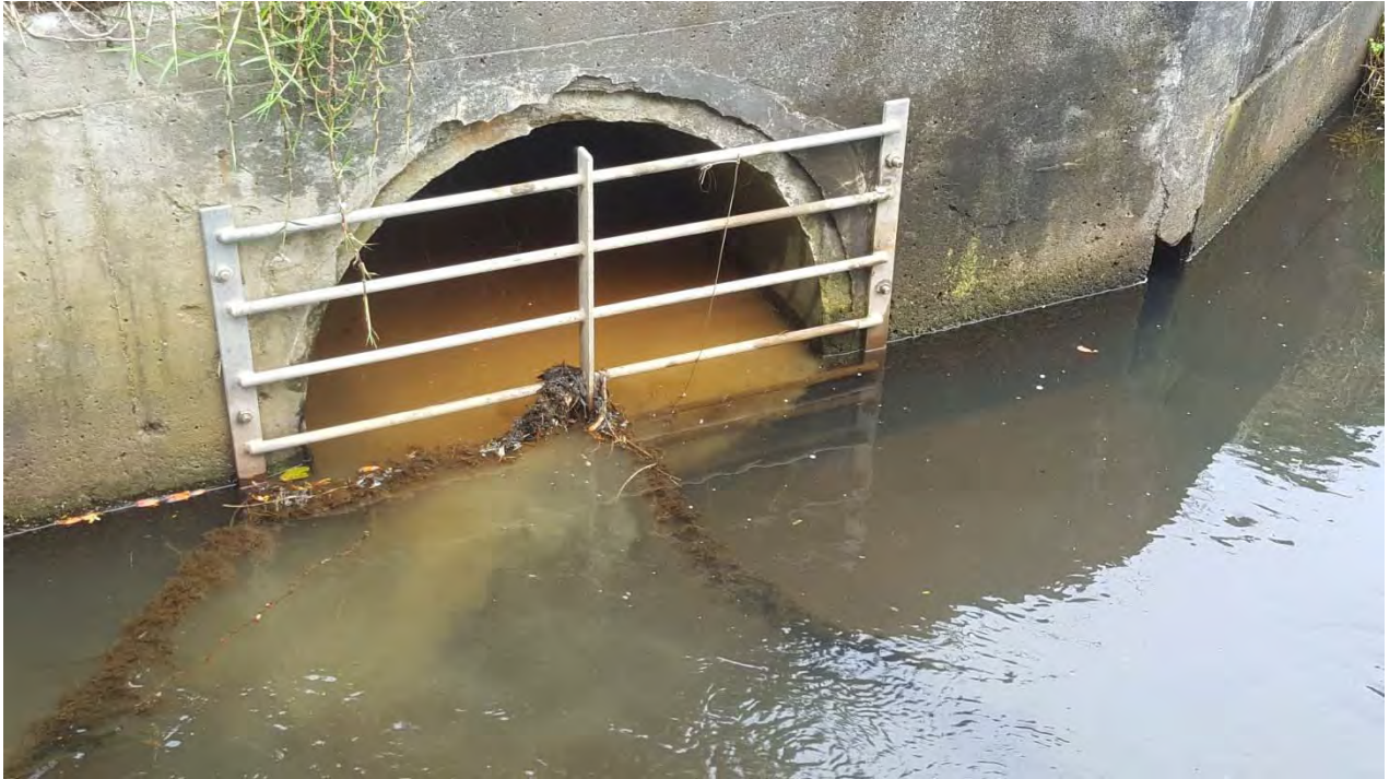
Figure 2 Light brown discharge from stormwater drain at time of survey
